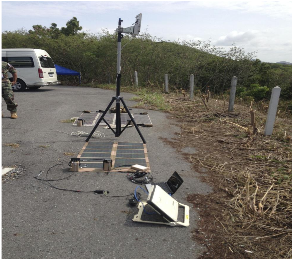
Figure 24. Hughes 9201 BGAN Terminal Connected to a WiMAX Antenna (from Crimson Viper 2013, Hat Yao, Thailand)
