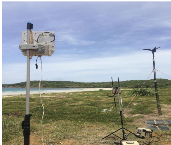
Figure 32. RENEWS with WiMAX and Wave Relay AP at C-IED Site
