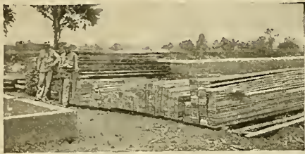
1 STARTING. "Honor Bill" material all measured and sawed at our factory by modern machinery ready to be speedily used. Watch the quick progress.
