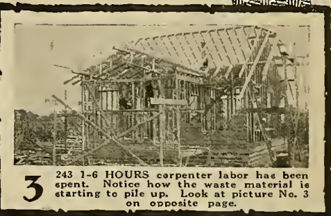
2 11 1/2 HOURS of carpenter labor on the material furnished in the ordinary way. Look at picture No. 2 on opposite page.
