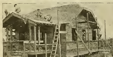
4 158½ HOURS carpenter labor—house all enclosed and under roof. You can be living in your "Honor Bill" home shortly after you place your order with us.
