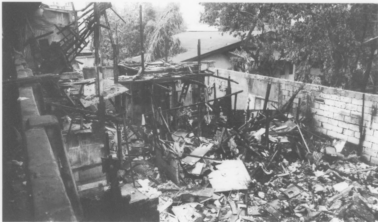
Above: The Buting Bridge fire left ruin in its wake. Below: Two young fire victims settle into their temporary housing.
