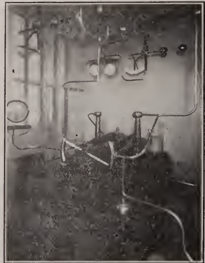
High voltage transformer with overhead system. (Author's equipment.)
