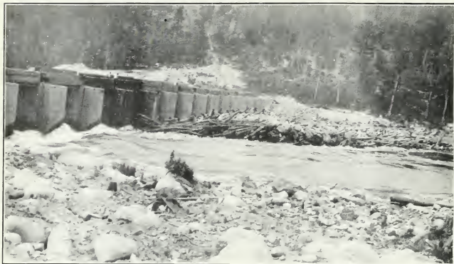
No. 1.—Timiskaming Dam. Ontario sluiceways, showing logs jammed against the piers, June, 1910, and swift flowing approach channel.
