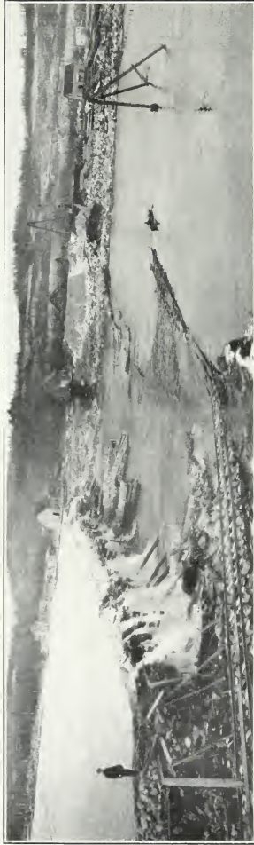
No. 6.—Timiskaming cofferdam, Quebec channel, Quebec channel, 3rd May—day before failure—lake surface elevation 581.50. The pit was flooded from below by Gordon Creek water several days before.
