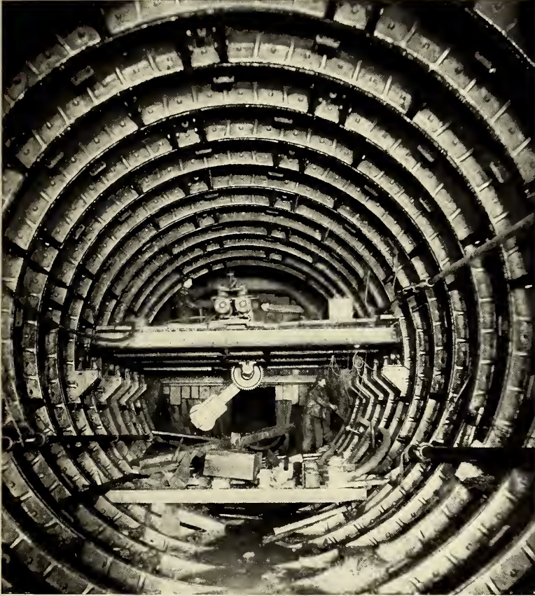
INSIDE THE TUNNEL, SHOWING THE "ERECTOR," BACK OF THE HORIZONTAL PLATFORM, RAISING A LINING PLATE TO POSITION.
