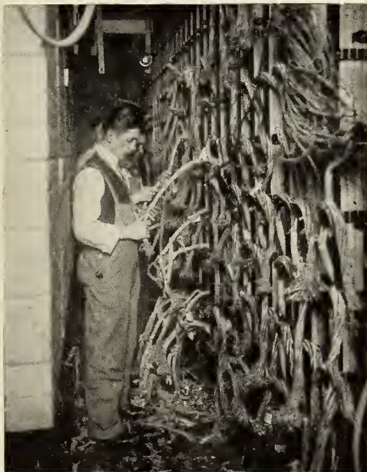
SORTING OUT A TANGLE OF WIRES AT THE BACK OF A DISTRIBUTING FRAME.
