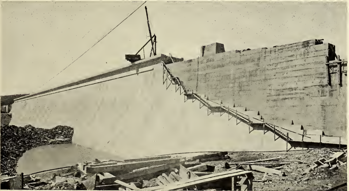
THE DOWN-STREAM FACE OF THE MASONRY PORTION OF THE OLIVE BRIDGE DAM.
