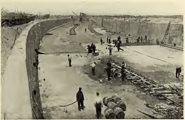
WATERPROOFING CONCRETE TROUGH WHICH IS TO CARRY THE AQUEDUCT WATER ACROSS IRONDEQUOIT CREEK.
