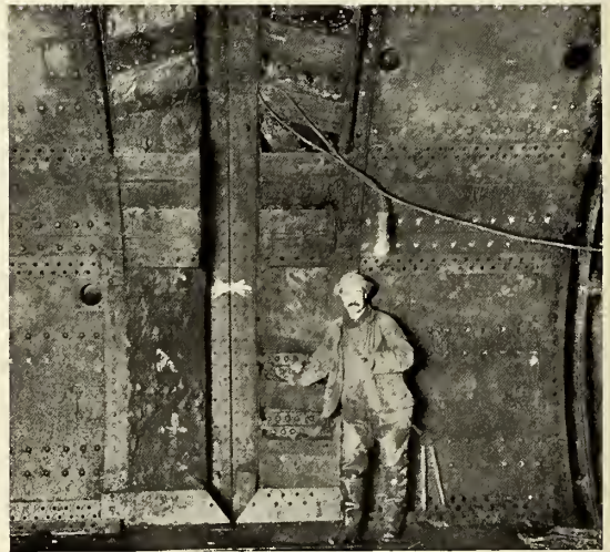
TWO SHIELDS, PUSHED FROM OPPOSITE SIDES OF THE RIVER, MEETING WITH A PERFECT FIT.
