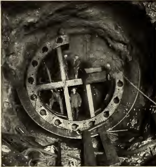
PUTTING UP A SHIELD WHERE THE TUNNEL IS ABOUT TO BREAK OUT OF THE ROCK.
