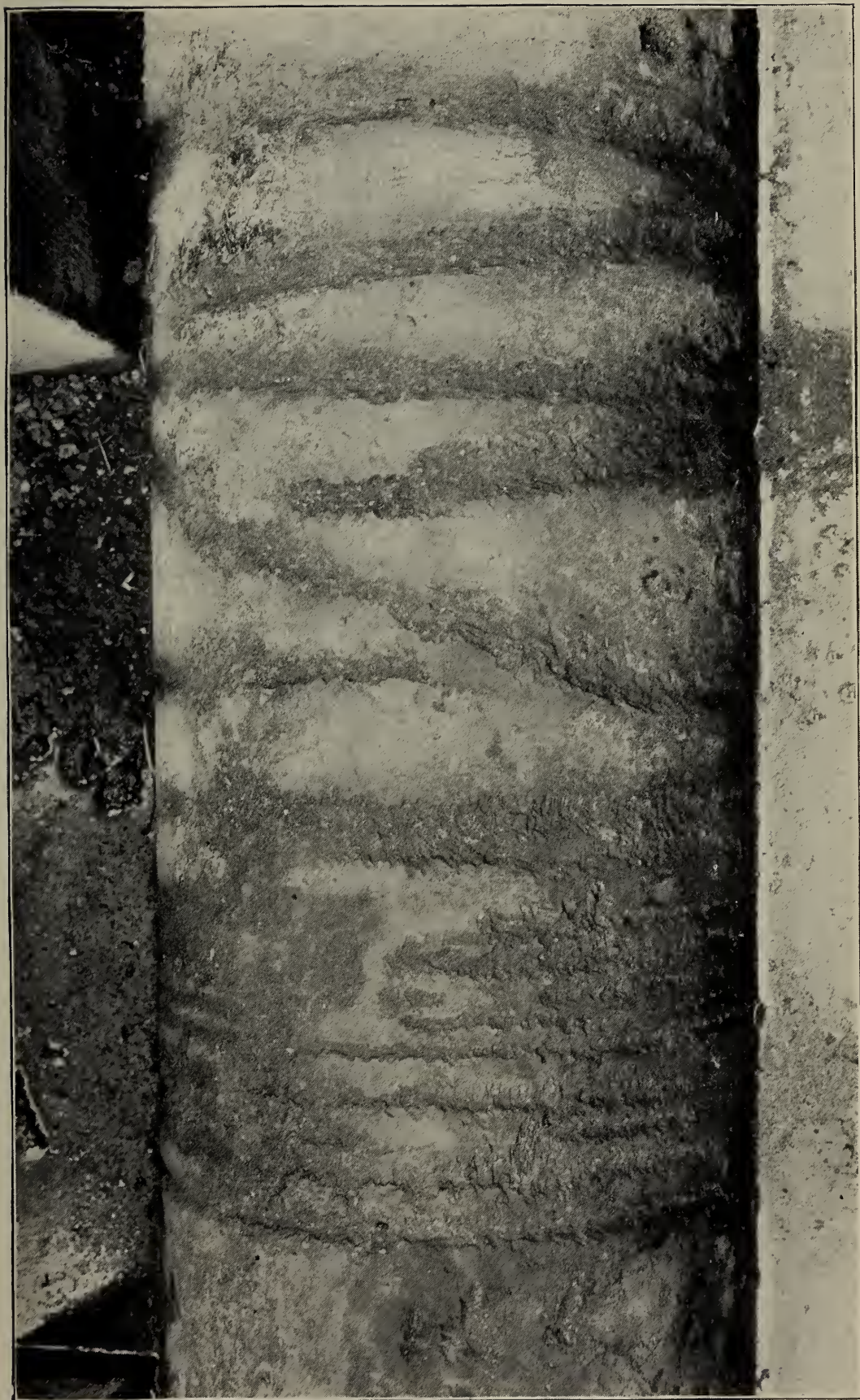
12-INCH PIPE IN WASHINGTON STREET IN LYNN, PITTED BY ELECTROLYSIS (REPLACED).
