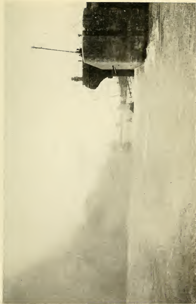
THE RIVER WINS: COLLAPSE OF A REGULATOR
