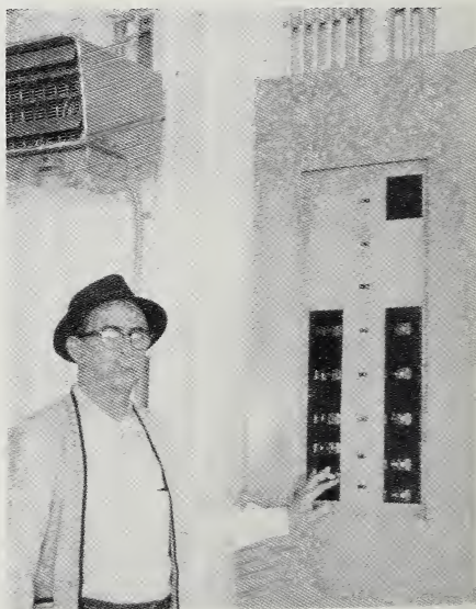
Mr. Allen at controls. Note quartz heating unit at upper left. In garage section, six of these units, hung from the ceiling, are used for heating and de-icing vehicles. Units range in size from 3,000 to 10,000 watts.
