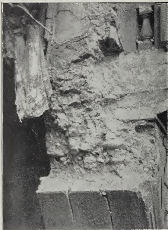
FIG. 7. Broken arch of the Palazzata showing rubble construction.
