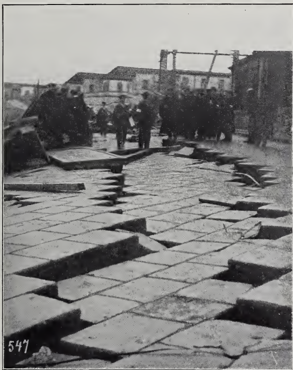
FIG. 4. Partial collapse of the embankment.
