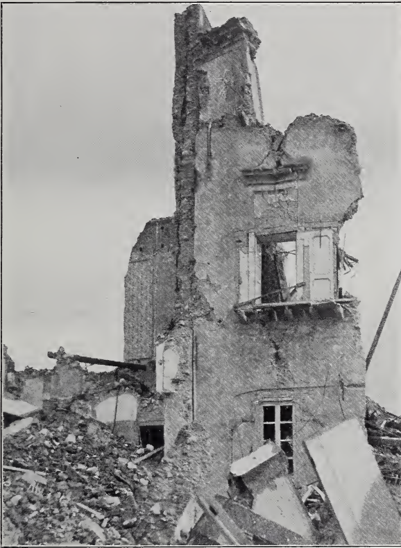
FIG. 8. Ruin of French Consulate. Walls fairly thick and well built but floors weak and house too high for this type of construction.
