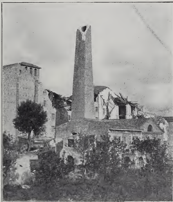
FIG. 10. Tall stack ; top snapped off and fallen S.S.W.
