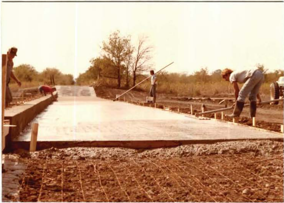
The construction of a low water crossing at the south end of Dever Pond Dike. (WRJ)
