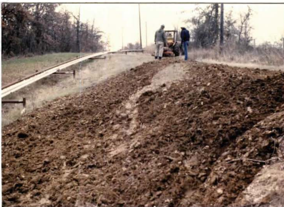
Treatment of salt contaminated soils by Shell Oil and Petromend (TM) crews. (WRJ)
