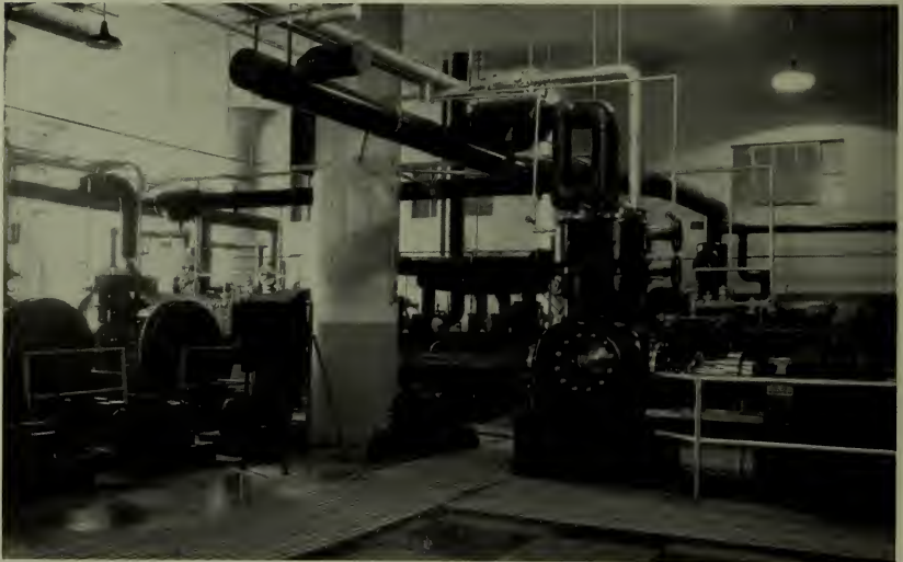
INTERIOR VIEW, STATE REFRIGERATION TERMINAL, SHOWING COMPRESSOR ROOM
