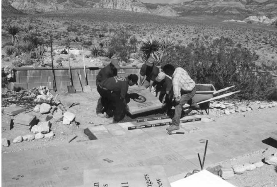
On National Public Lands Day 2001, BLM and two partner groups—the Friends of Red Rock Canyon and the Red Rock Canyon Interpretive Association—dedicated a memorial to the victims of September 11. The 300-pound memorial stones are made of metaquartzite, which was excavated from a quarry near Goodsprings, NV.
