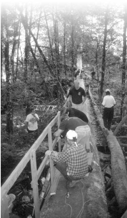
National Public Lands Day volunteers in the Eugene (OR) District worked to construct a footbridge at the McGowan Creek Environmental Education Area, northeast of Springfield.
