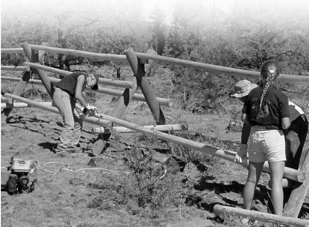
National Public Lands Day 2001 was a busy day in Oregon. At the Gerber Recreation Area near Klamath Falls, volunteers were involved in many projects, including buck-and-pole fence construction.
