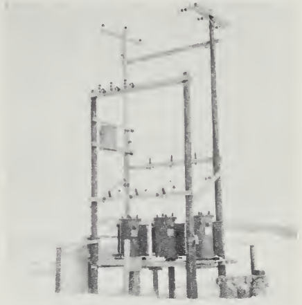
Three 250 KVA transformers enable quarry to meet increasing demands.
