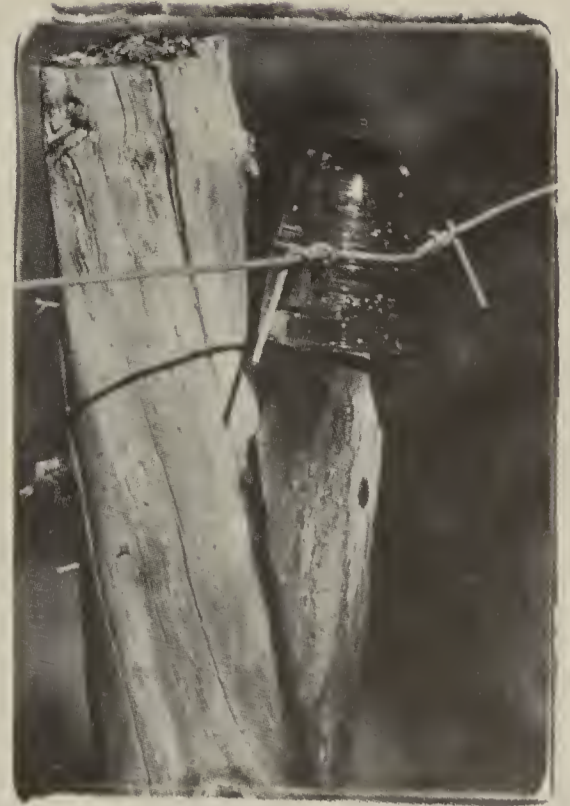
Insulators on WAMCATS line. (BLM Photo)
