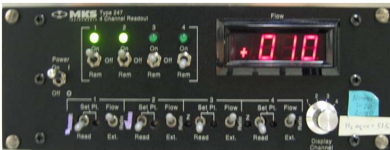
Figure A-13. Mass-flow Controller.
