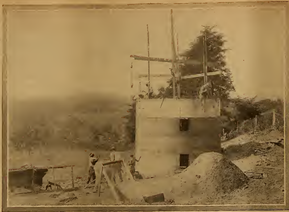
A scene from the film of U. S. Department of Agriculture entitled "Construction of a Concrete Silo"
