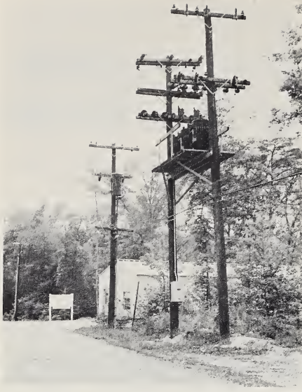
Transformer and lines leading to Blossom Point's 150 KVA substation of Southern Maryland Electric.
