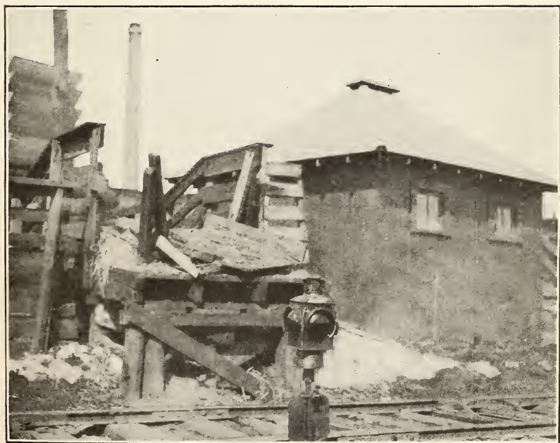
FIG. 2.—A DILAPIDATED LOADING AND UNLOADING CHUTE.
