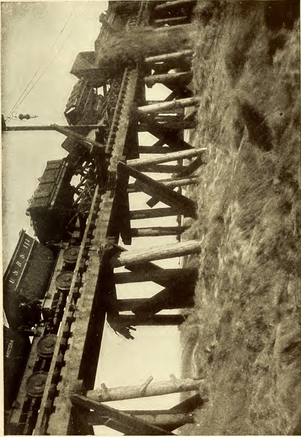
CLOSING COLORADO RIVER DURING CONSTRUCTION OF LAGUNA DAM, YUMA PROJECT, ARIZONA-CALIFORNIA Nearly 72,000 cubic yards of material were dumped into the stream before the closure was effected. The Laguna dam now completed is 4,780 feet long, 19 feet high, and weighs 600,000 tons
