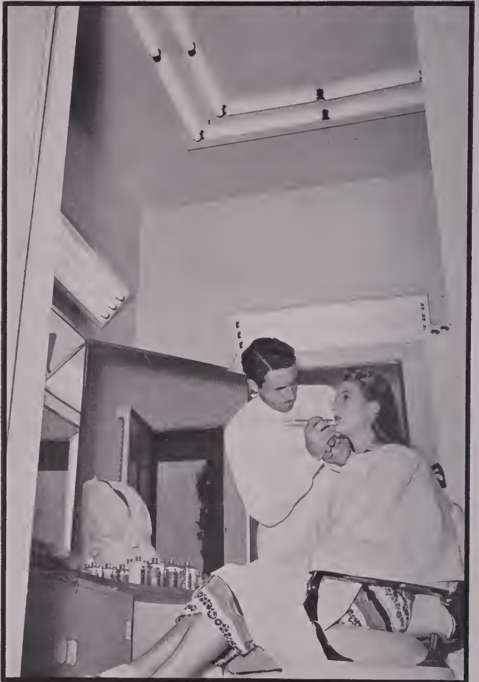
This installation was designed and constructed by W.T. Strohm, Chief Engineer of 20th Century-Fox. It employs twenty-eight of the new Daylight Fluorescent MAZDA lamps . . . to provide glareless light, of daylight quality. Clay Campbell, Director of Make-Up for 20th Century-Fox, is shown applying make-up to Binnie Barnes, popular screen artist, for her latest picture, "WIFE, HUSBAND AND FRIEND."
