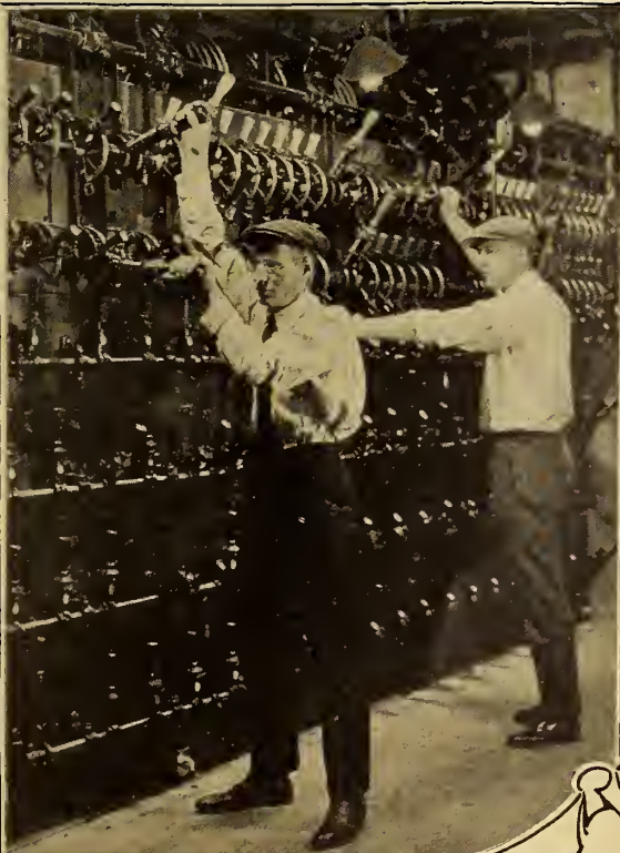
Pre-set Switchboard. EASTMAN THEATRE - ROCHESTER N. Y.
