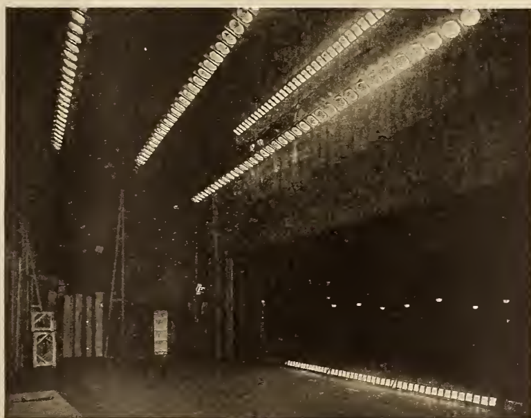
FIG. 5 Individual Aluminum Finish Steel Angle Reflectors with 100-watt Mazda C Lamps are Used as Border Units on this Stage. The color screens have been removed. Three circuits are provided in the borders and four in the concert border. Footlights are similar in character but more closely spaced
