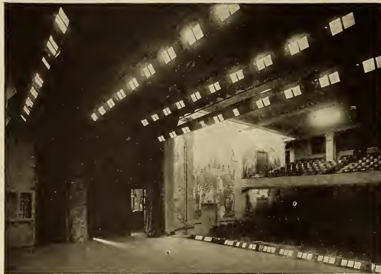
View of Stage with Modern Type of Footlights and Borders. Individual reflectors of metal painted white are used with gelatin color screens. 100-watt lamps are placed on 6-in. centers. Four circuits are provided in both foots and borders
