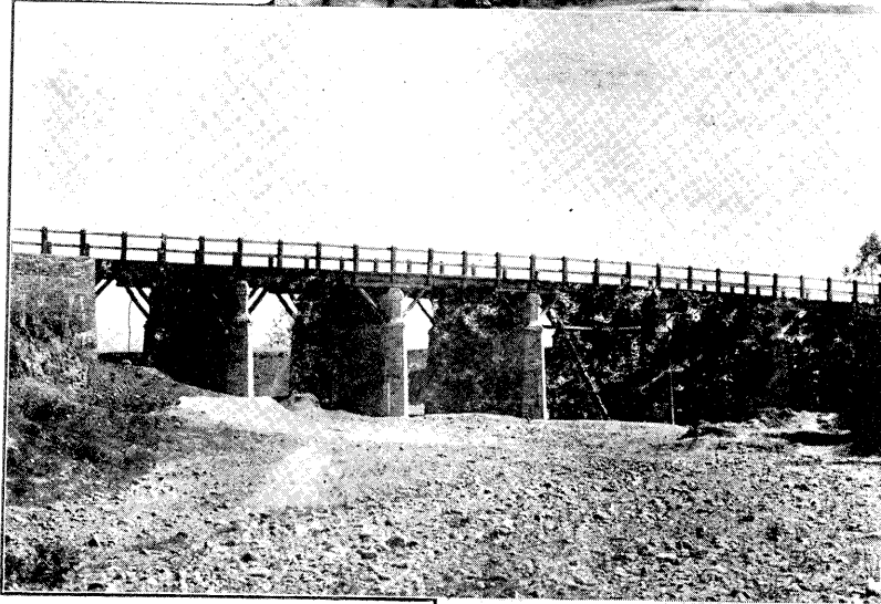
← 河南洛潼公路后莊河橋 THE HOU-CHUANG-HO BRIDGE ON THE LOYANG- TUNGKUAN HIGHWAY IN HONAN PROVINCE
