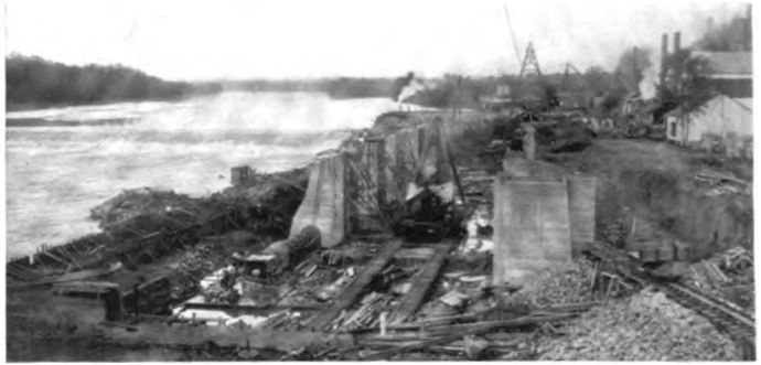
VIEW OF OPERATIONS AT LOCK 4 ON THE COOSA-ALABAMA RIVER, SHOWING COMPLETED DAM AND WORK IN PROGRESS ON THE WALLS OF THE LOCK.
