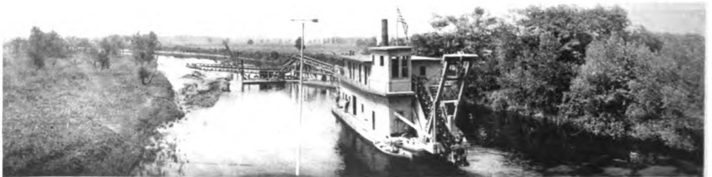
THE APPARATUS THAT CLEARS THE WAY TYPE OF U. S. ARMY ENGINEER CONVEYER CHANNEL DREDGE EMPLOYED IN SWAMP DRAINAGE OPERATIONS
