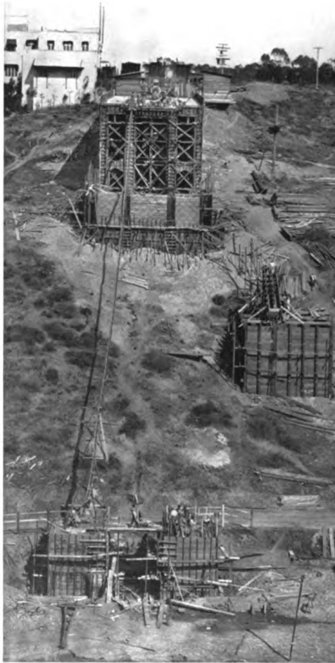
ERECTING A 900-FOOT BRIDGE TO SPAN A PICTURESQUE CANYON IN EXPOSITION PARK, WHICH IS TO BE PERMANENTLY MAINTAINED BY THE MUNICIPALITY
