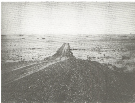
FIGURE 1-18. TEMPORARY ROAD BUILT FOR HAULING DRILLING EQUIPMENT FROM ONE SITE TO ANOTHER.
