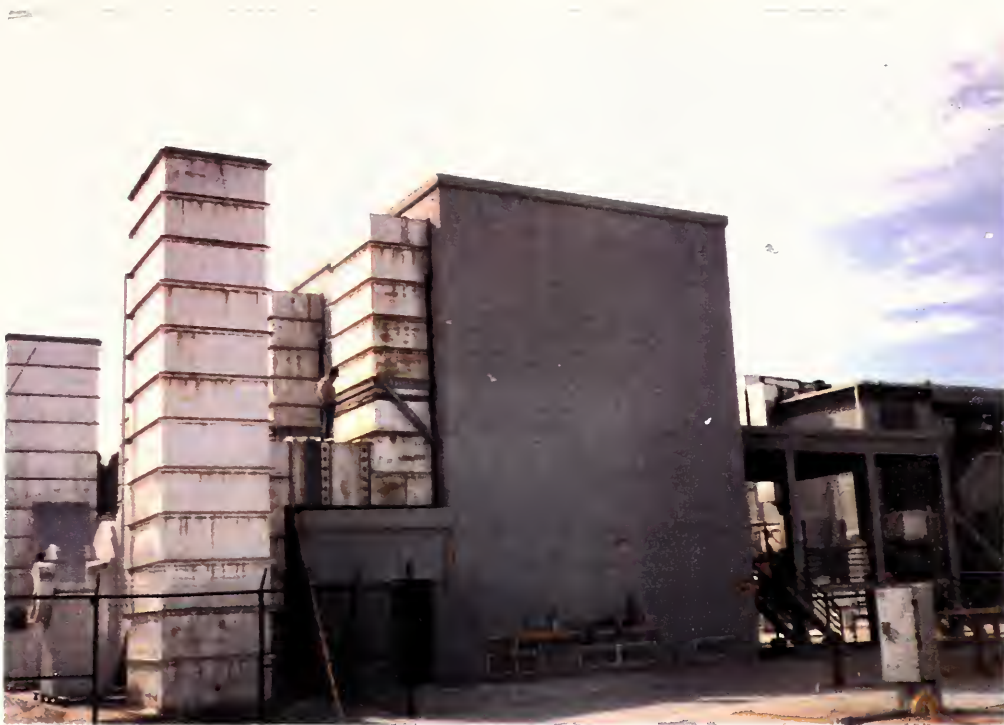
Figure 14A - 19F3-B4 Ventilation Ducts
