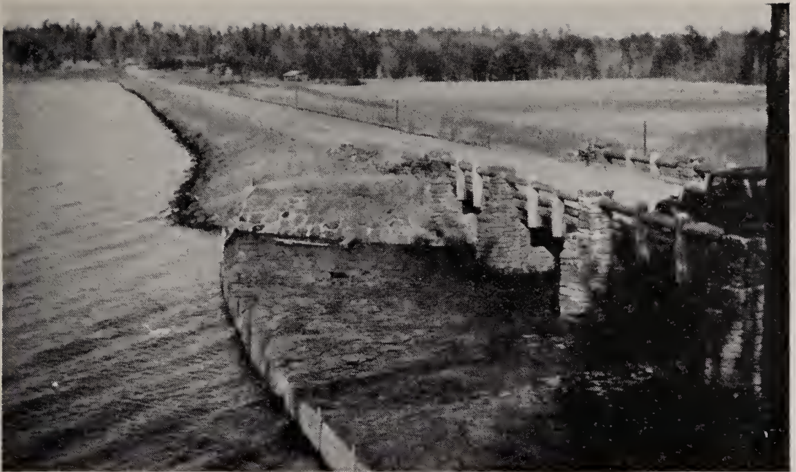
A view of Choctaw Dam and Lake, with the spillway in the foreground, and the roadway and bridge which contribute to the recreational development
