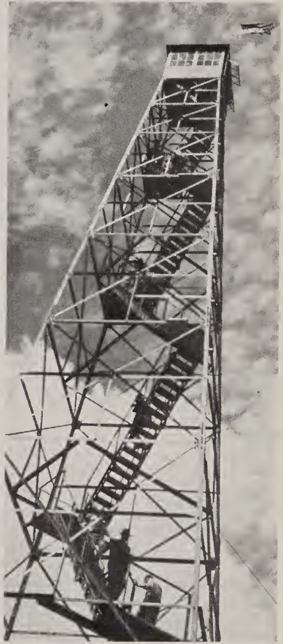
One of the project's two giant fire towers that are helping to make the area's trees a permanent asset
