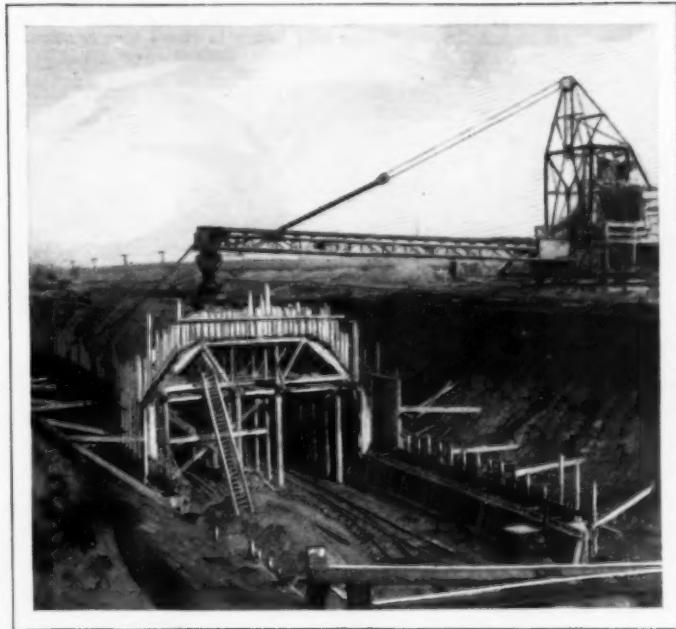
Building a Subway in Berlin; the Tunnel Sides and Top Are Constructed of Steel and Concrete After Channel Is Excavated
