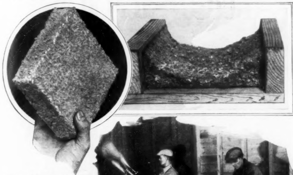
Section Cut from Inch-Thick Paper Insulation; a Section in Place between Studding, and the Paper Blower and Nozzle in Action; the Two Fine Streams are Atomized Water Glass for Binder
