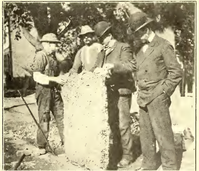
BOSTON ELEVATED RAILWAY, HIGH STREET, MEDFORD, SHOWING THE THICKNESS AND UNDER SIDE OF A SECTION OF THE BITULITHIC PAVEMENT, CUT FROM BETWEEN THE TRACKS TO INSTALL A CATCH-BASIN INLET
