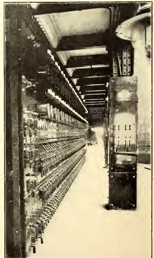
FIG. 35.—SWITCHBOARD FOR HIGH-TENSION FEEDERS, CHELSEA POWER STATION
