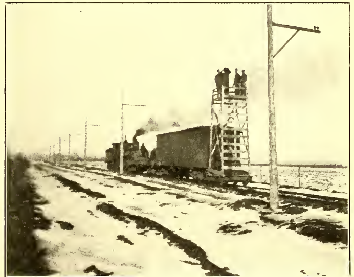
METHOD OF STRINGING OVERHEAD WIRES ON THE PONTIAC SINGLE-PHASE LINE, USING A CONSTRUCTION LOCOMOTIVE
