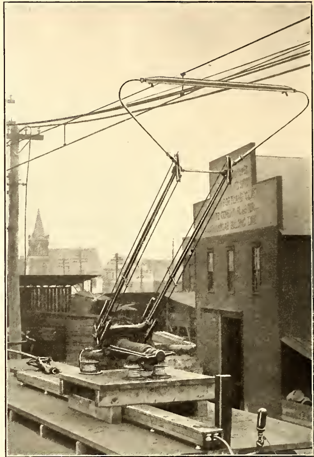
BOW TROLLEY CONNECTED TO BASE MOUNTED ON INSULATORS
