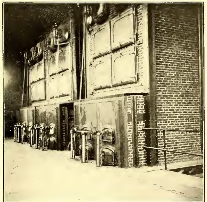
BOILER ROOM, SHOWING OIL BURNERS
