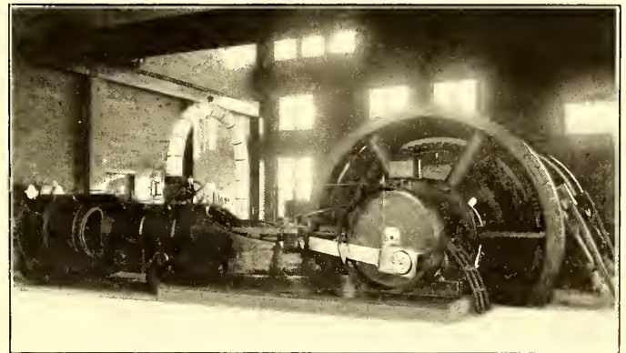
MAIN GENERATOR AND ENGINE IN POWER STATION
