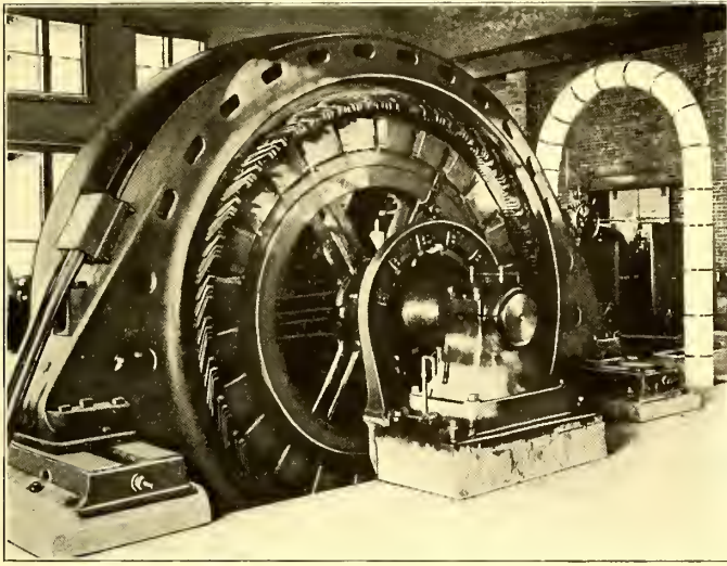
ONE OF THE GENERATORS
