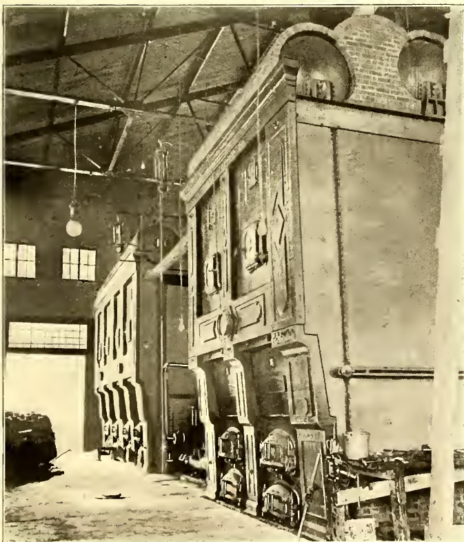
A VIEW IN THE BOILER ROOM
