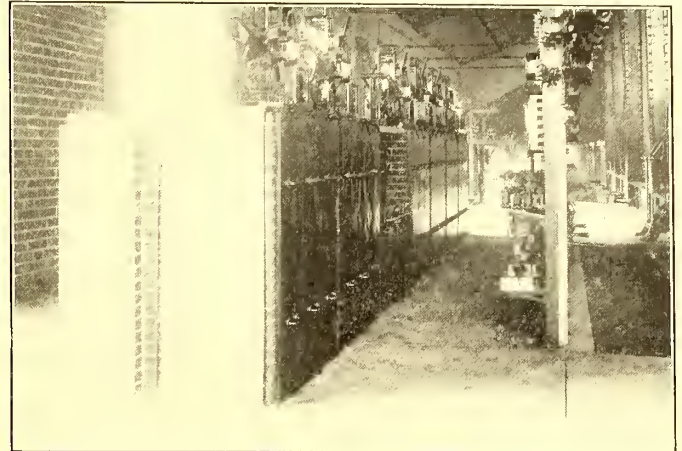
FIG. 3.—OVERLOAD RELAYS AND HIGH-TENSION OIL SWITCHES
