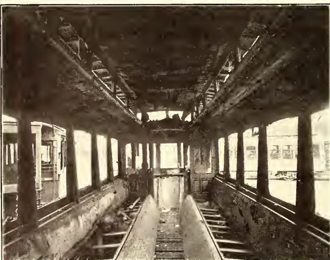
CAR IN TEST NO. 3—AFTER THE FIRE
