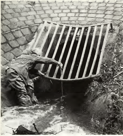
Fig. 1. Upstream end of the culvert conveying water from Monbulk Creek through the flood retarding basin embankment.
