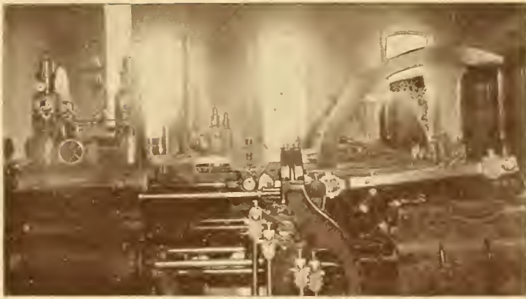
INTERIOR PUMPING STATION—ASHLAND WATER CO.
