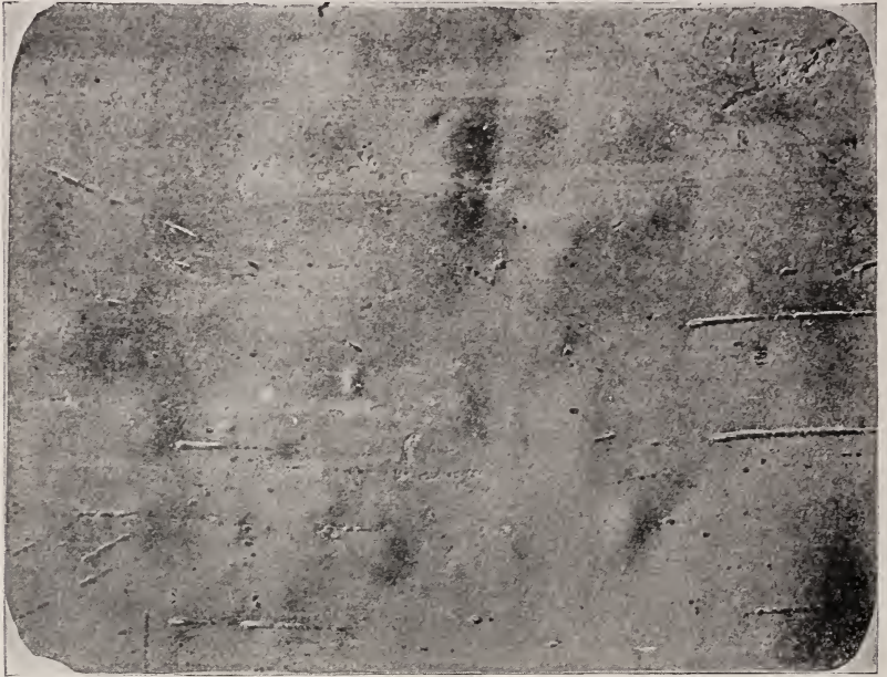
FIG. 49.— Appearance of the exposed surface of corroded tinned copper sheathing used for roofing purposes. \times 1
