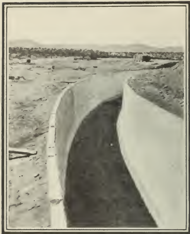
A VIEW OF THE CONDUIT IN THE DESERT, LINED AND READY FOR COVER
