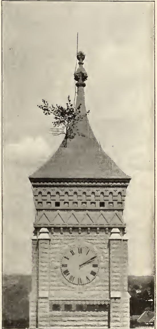
THE TREE GROWING ON THE COURT-HOUSE TOWER.
