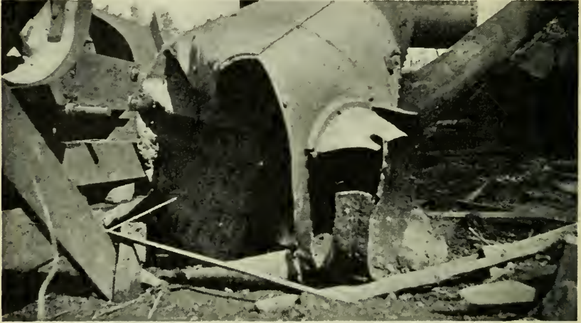
Figure 2. Aftermath of corrosion around the crown bolts of a locomotive type boiler.
