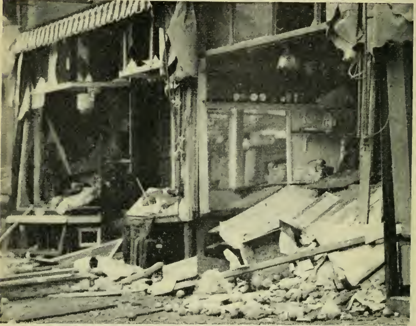
A cast iron boiler explosion on November 18, 1935, injured four persons and wrought damage estimated at $10,000 to these stores.
