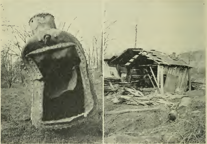
Left:—Boiler after 300 ft. journey. Right:—The shattered engine house where the eight persons who were killed or injured had gathered.
