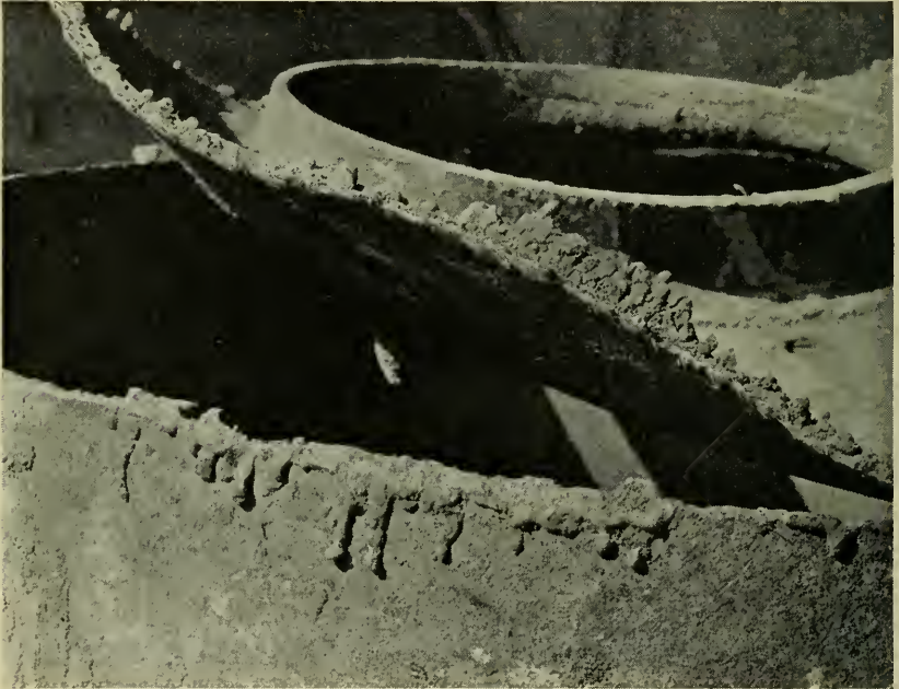
Close-up view of welded seam failure.
