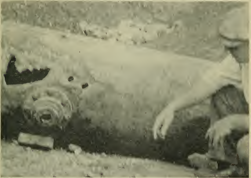
Extreme external corrosion in a buried blow-off tank. Conditions with respect to this form of wasting away are particularly serious whenever a vessel is installed underground.
