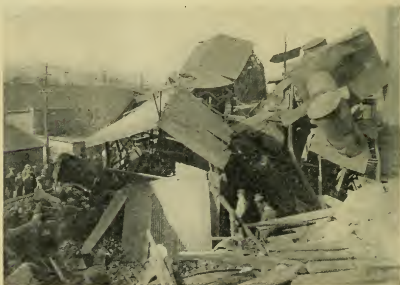
After a corroded mud drum head blew out at an Indiana paper mill.
