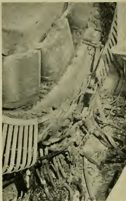
Windings and leads damaged by short-circuiting and fire
