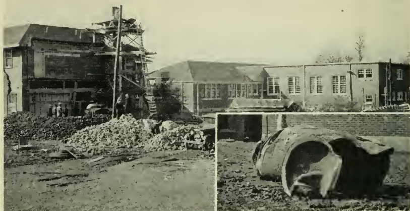
Repairing damage after explosion. Observe the 3' hole (boarded up) in brick wall of gymnasium, extreme right of picture by small double windows. Inset—Remains of tank showing reversed minus head.
