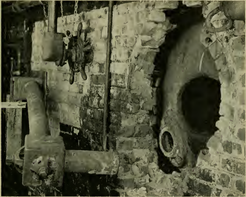
Circulating tube which pulled out of drum. Prompt drawing of the fire prevented serious overheating of the draining boiler.
