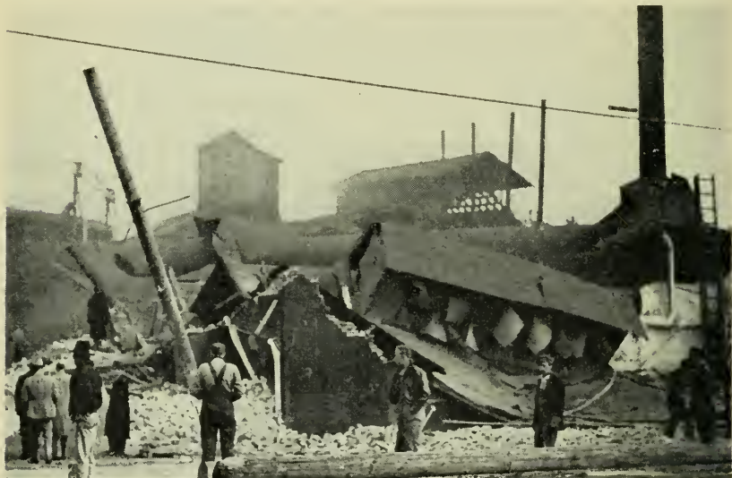
Result of external corrosion of a blank head in a bent tube type boiler.
