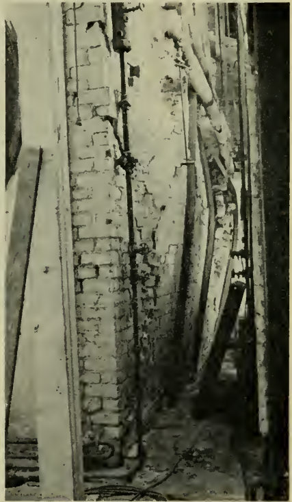
View of right side wall of No. 2 boiler showing the damaged setting. The boiler is 72" in diameter and 16' long of the horizontal return tubular type.
