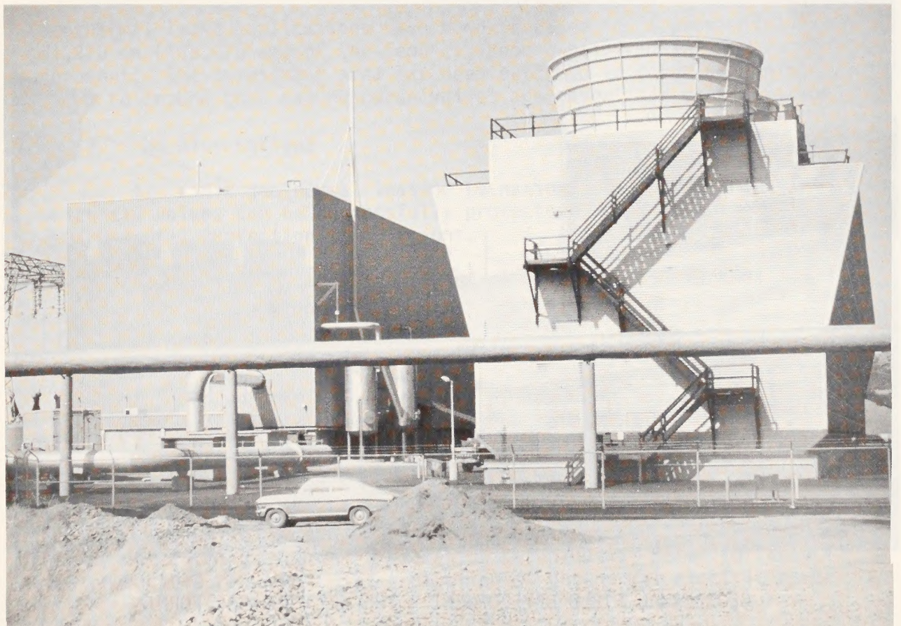
POWER PLANT (110 MW) AT THE GEYSERS, CALIFORNIA
