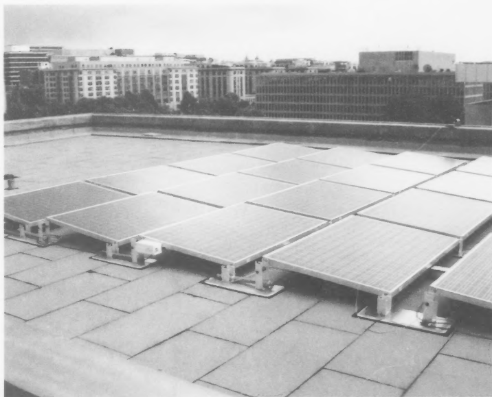
New solar panels grace the roof of the Harry S Truman Building.
