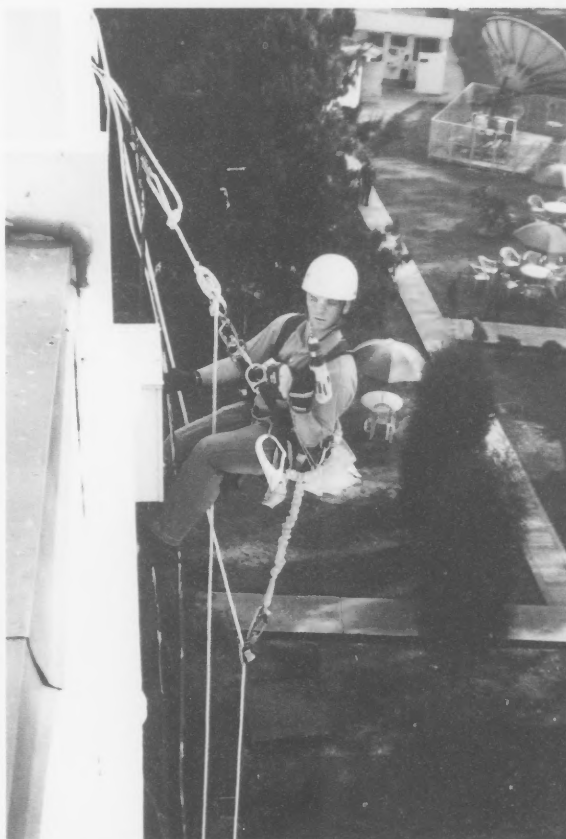
Contractor Brad Raupp uses his rappelling skills during the WEXTEL installation in Kathmandu.
