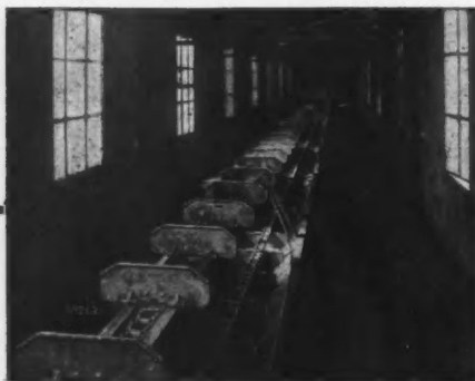
Scraper Conveyer Handling Coal Over Bunkers in Boiler House
