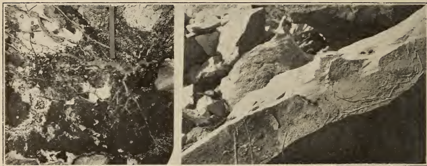
FIG. 9. Cracks in chert filled with limestone.
