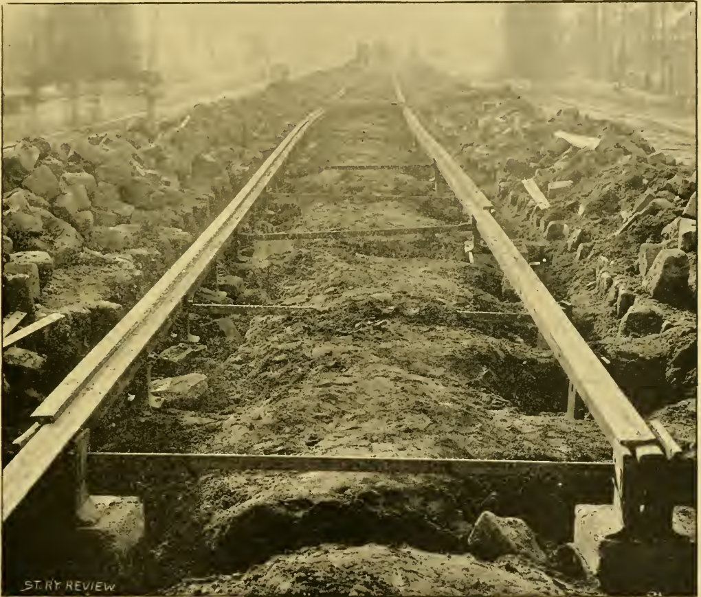
LAYING THE DUPLEX RAILWAY TRACK SYSTEM ON FOURTH AVENUE, NEW YORK CITY.
