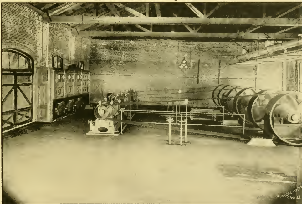
SHORT GENERATORS—POWER HOUSE OF JAMESTOWN, N. Y., ELECTRIC RAILWAY.
