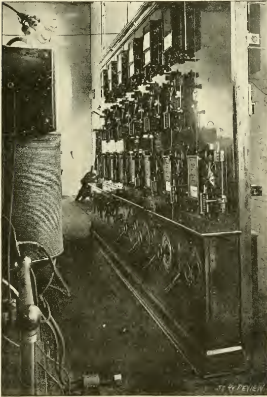
SWITCH BOARD—BROADWAY AND NEWBURG.
