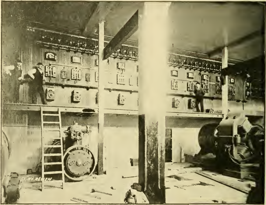
THE SWITCH BOARD.
