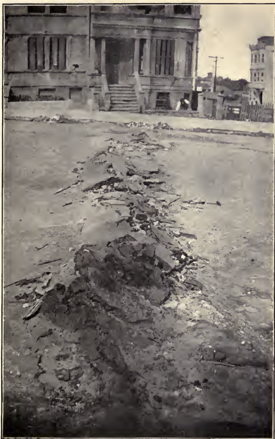
From a Stereograph, Copyright, 1906, by Underwood & Underwood A SAN FRANCISCO PAVEMENT TORN BY THE EARTHQUAKE
