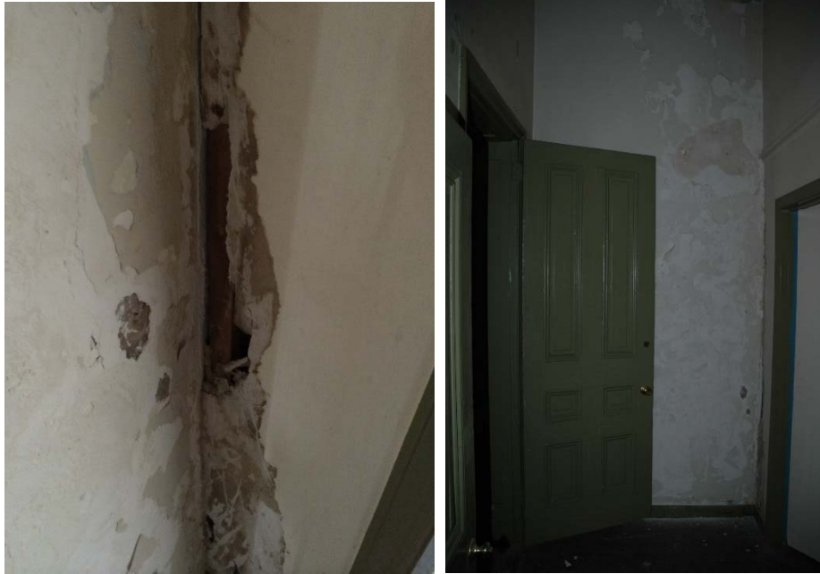
Figure 1.5-30: View of plaster damage in southwest corner (left) and south wall (right) of Room 107.
