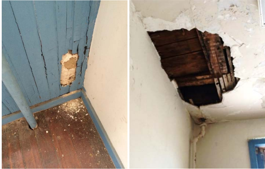
Figure 1.5-31: Detail view of wood wainscot damage in Room 108. Note plaster wall damage behind the wainscot and mechanical system penetration at wood floor (right). Detail view of plaster ceiling damage in Room 108 (left).
