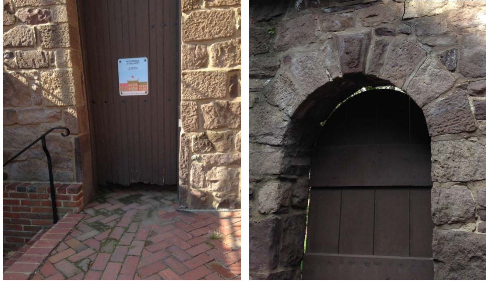
Figure 1.5-13: (Left) The board-and-batten door to the access ramp displays moderate deterioration at bottom edge due to water penetration through the end grain. (Right) The board-and-batten door at the courtyard wall is in good condition despite minor deterioration at the bottom edge.
