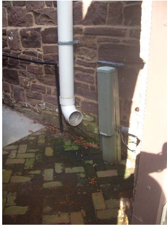
Figure 1.5-4: The brick paving under the downspout is extremely slippery due to a heavy build-up of algae and constitutes a safety hazard.
