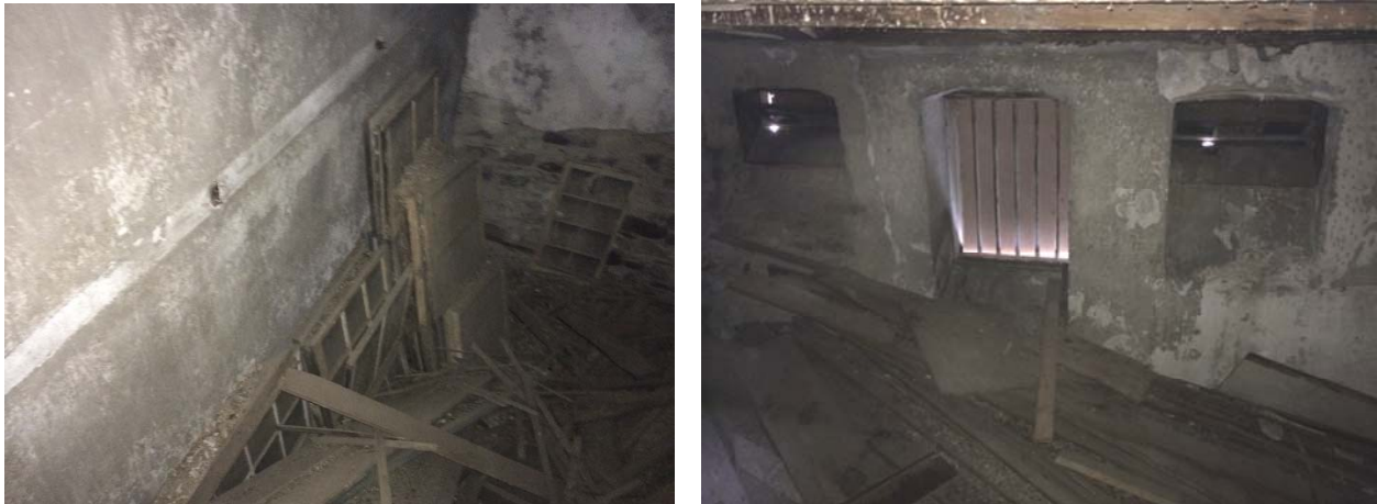
Figure 1.3-46: View of Room 211 looking northwest (left), view of Room 211 looking east at wall, door and windows (right).
