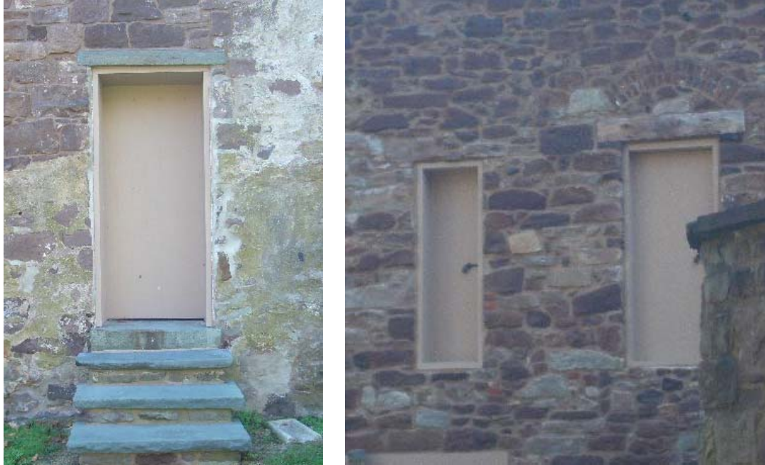
Figure 1.5-12: (Left) The existing wood door leading into the old cell area consists of a board and batten door in a simple wood frame. The door may be opened from the inside only. (Right) The doors to the second-story prison cells are similarly constructed but with locking hardware on the exterior.
