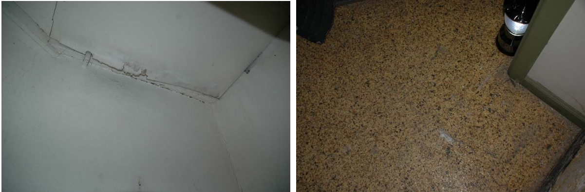
Figure 1.5-35: View of cracking at ceiling (left) and 20 th century epoxy flooring (right) in Room 112.
