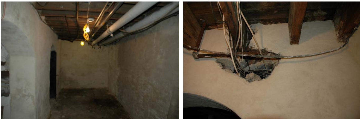
Figure 1.5-17: Views of loose building systems (left) and plaster damage at penetrations (right) in Room 002.
