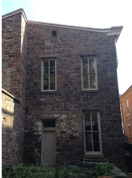
Figure 1.3-13: The windows on the west façade are rectangular rather than arched though the hierarchy of window heights is consistent with that observed on the east façade. The lintels of the first and second-story windows differ.
