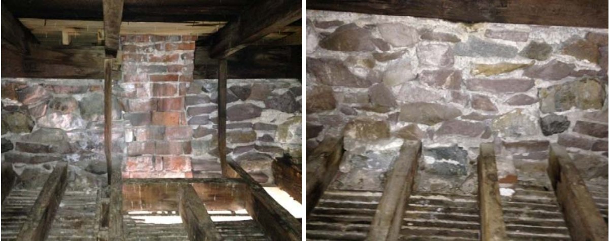
Figure 1.2-56: (Left) Framed opening in attic floor for the missing fireplace centered on the south wall of the southwest room. (Right) Attic joists bearing on chimney mass of newer fireplace in Room 207. No framed floor or roof opening is evident at this location.
