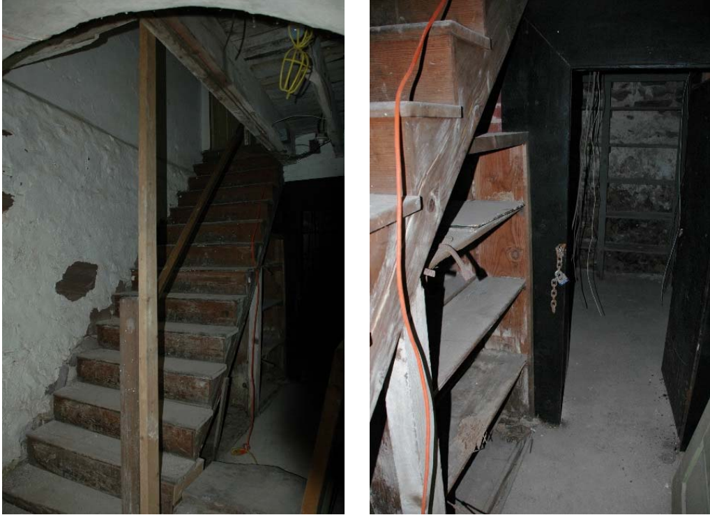
Figure 1.3-19: Views of Room 004 looking south at stair (left) and looking south down corridor to Room 005 (right).
