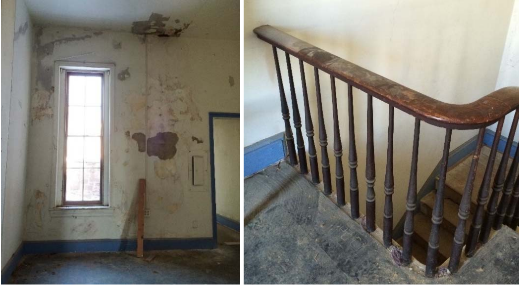
Figure 1.5-44: North view of plaster damage in Room 205 (left). Detail view of second floor stair balustrade in Room 205 (right).
