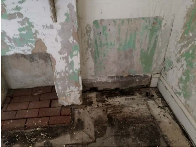
Figure 1.5-46: Detail view of plaster and wood base damage at Room 207 (left).
