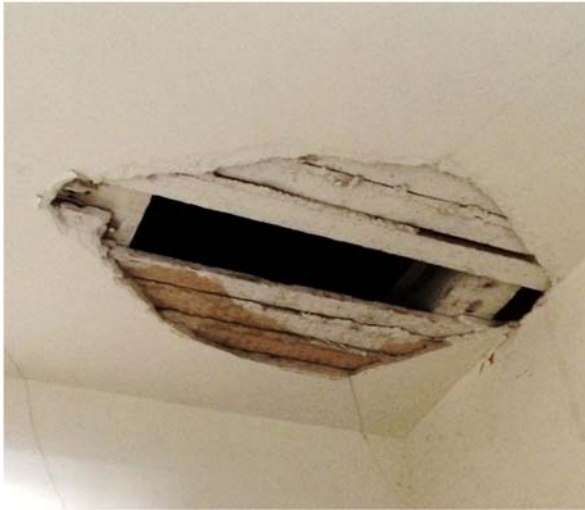
Figure 1.5-45: Detail views of damaged and missing plaster in Room 206 (left).
