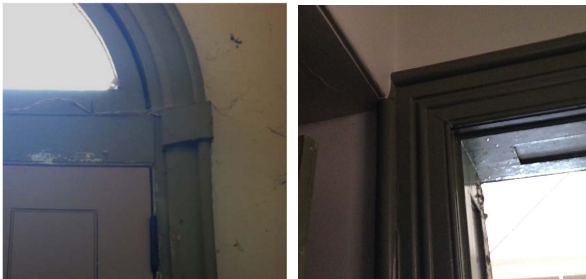
Figure 1.2.25: (Left) The door trim molding at the front entrance doors is simpler in profile than that seen at other openings (Right) which suggests an earlier date in keeping with the late Greek Revival of the mid-19 th century rather than the late 19 th -century Victorian period. The paneled jamb seen at right is simpler and consistent with the front door trim and is likely original to 1857.
