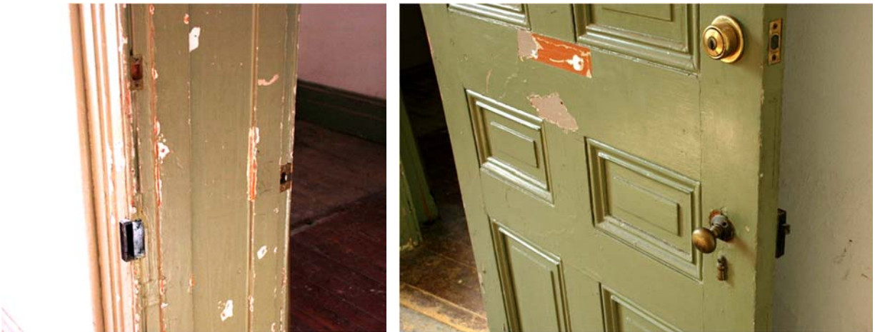
Figure 1.5-24: Detail view of damage and multiple hardware campaigns at jamb and door at Room 101 (top left and right).
