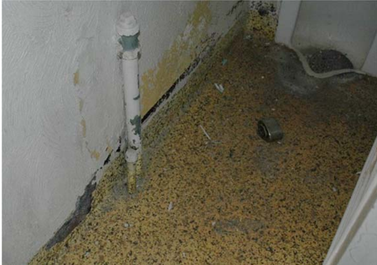
Figure 1.5-36: Detail view of epoxy floor and damaged integral base in Room 113.
