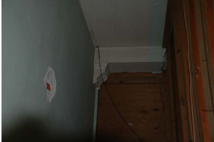
Figure 1.5-29: View of plaster bracket and plaster damage at west wall in Room 106.
