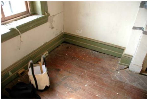
Figure 1.5-26: Detail view of original marble mantel damage in Room 103. Note plaster damage where it abuts mantel (top left). Detail view of hinge at Door 2/103 (top right). Detail view of flooring deterioration at southeast corner of Room 103. Gap between floor and wood base indicates floor sagging. Sagging has resulted in cracking at the fireplace hearth.
