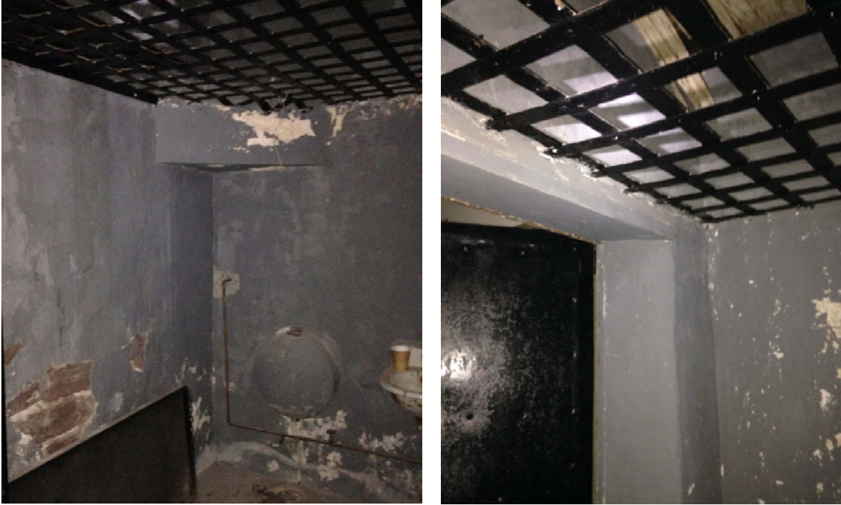
Figure 1.2.66: (Left) The cells in Rooms 112-114 are enclosed by a combination of parged masonry walls and iron grates salvaged from a Wilmington prison and installed in 1916. (Right) The existing door in opening 1/112 is. This door, a paneled wood door faced with plywood or similar material, would not have been suitable when this was a detention area and would have been installed later.
