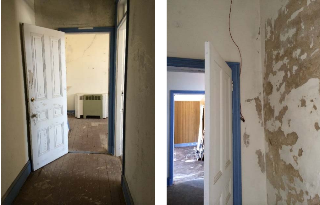
Figure 1.3-39: Views of Room 203 looking north with Room 201 beyond (left) and detail view of plaster damage at west wall (right).
