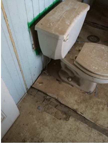
Figure 1.5-48: Detail view of modern sheet flooring over wood flooring in Room 209 (left).
