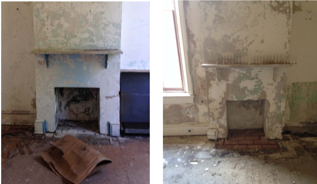
Figure 1.2.57: (Left) The new fireplace in Room 208 was eventually replaced by radiators, seen at right. (Right) The subdivision of the southwest room left Room 207 without any window. The window visible at left was added (or perhaps relocated) to provide light and air to the room.
