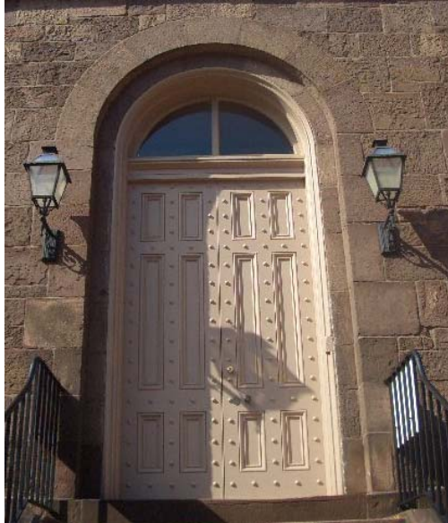
Figure 1.5-10: The existing doors were reproduced from the originals and are in good condition. The glass transom is almost certainly a replacement.
