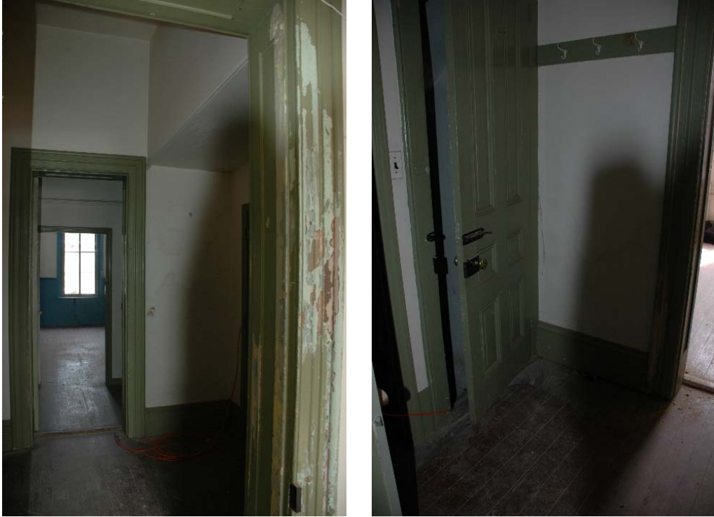
Figure 1.3-26: View of Room 105 looking west with Rooms 107 and 108 beyond (left) and looking northeast to door to basement stair (right).
