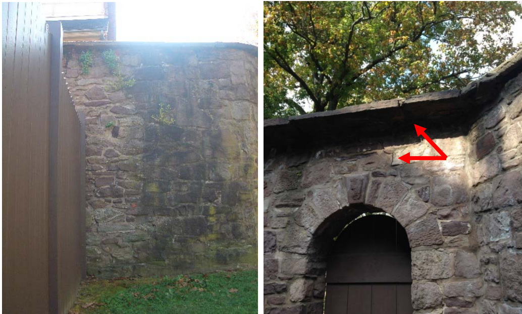
Figure 1.5-6: (Left) The heavy biological staining on the east face of the courtyard wall is caused by water entering through the coping joint above. (Right) Cracking observed at the gate arch is aggravated by moisture from the open joint above.
