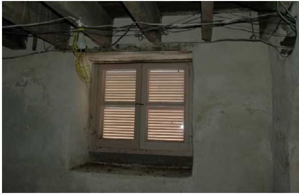
Figure 1.5-16: Detail views of plaster deterioration at west chimney support in Room 001 (top) and detail view of Window 001 in Room 001 (bottom).
