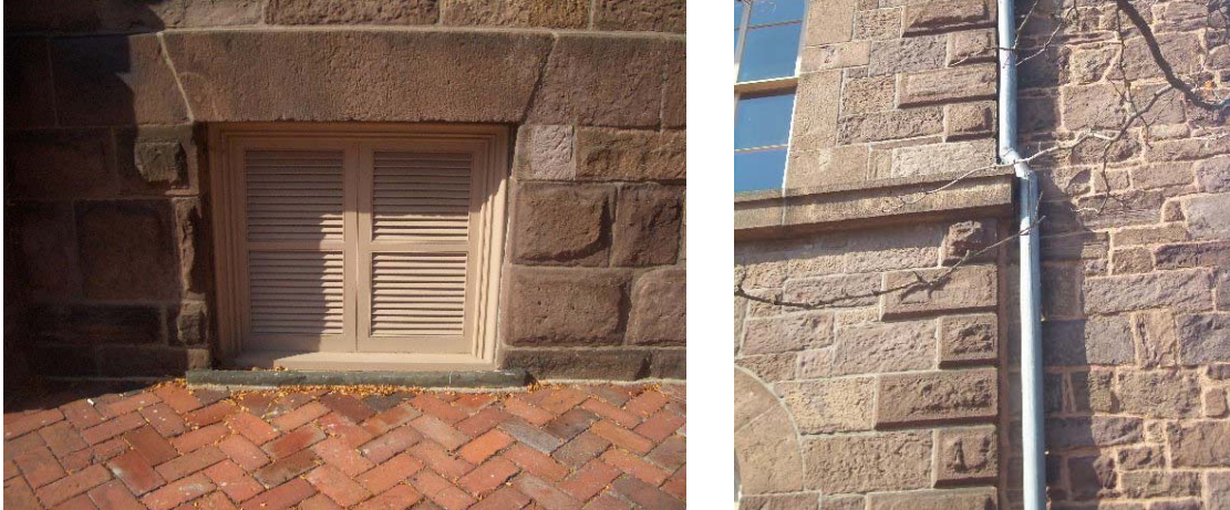
Figure 1.3-4: (Left) Rusticated masonry defines the foundation below the water table. (Right) Rusticated quoins define the corners of the otherwise smooth planes of the upper stories.
