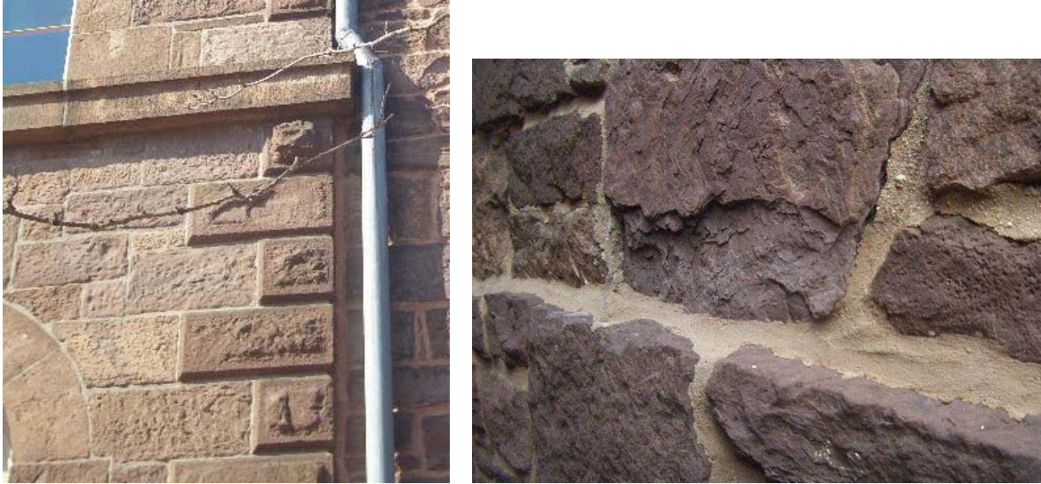
Figure 1.5-5: (Left) The ashlar stone used on the east façade is uniformly grained and properly bedded. It remains in very good condition. The rubble stone is less uniform and some isolated units exhibit significant delamination.
