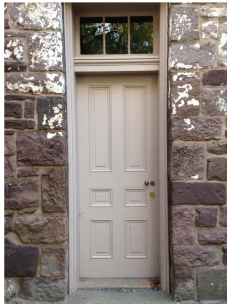
Figure 1.3-9: The west and south doorways are extremely similar. However, it seems unlikely that the west doorway shown above is original.
