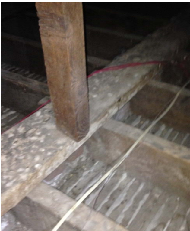
Figure 1.2-21: The fact that the post supporting the north valley of the front gable does not land on the bearing wall suggests strongly that the brick bearing wall is from an earlier structure. The post bears instead on a recycled floor joist a few inches away from the masonry that should be supporting it.
