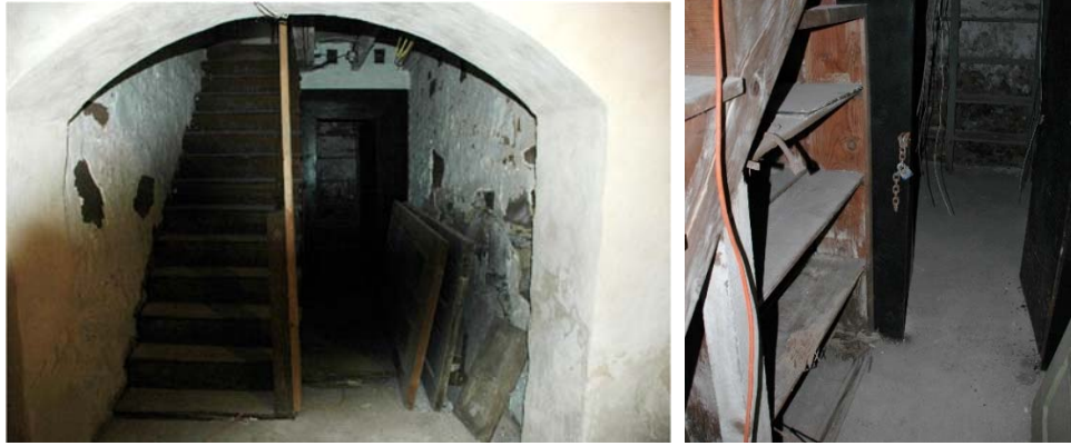
Figure 1.5-19: View of missing plaster (left) and under-stair shelving (right) in Room 004.
