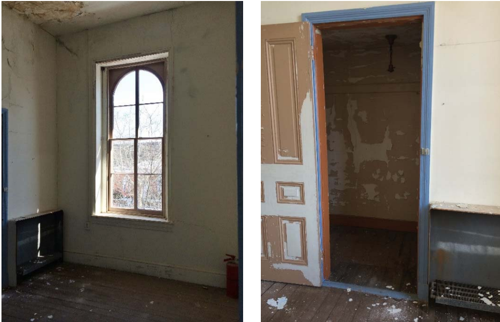
Figure 1.3-37: Views of Room 201 looking northeast (left) and looking east at original closet (right).
