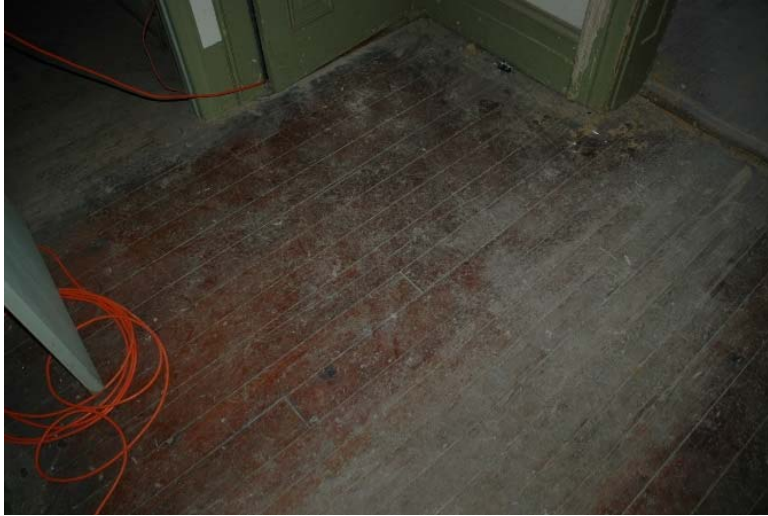
Figure 1.5-28: View of floor wear in Room 105. Note more serious wear at flooring near the east door in the upper right corner.
