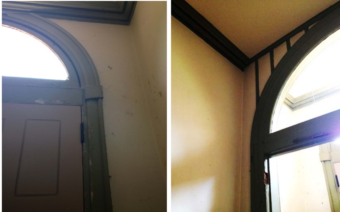
Figure 1.2.24 (Left) The trim on the arched transom collides with the run plaster cornice at the east end of the center hall. The awkward transition suggests that Sloan was trying to enlarge the door opening within the confines of existing second-floor framing. The trim on this door is a simple profile with a narrow backband; (Right) The partition forming the vestibule is a later addition and the complex trim profile with beaded edge, ogee molding and backband is consistent with a late 19 th -century date.
