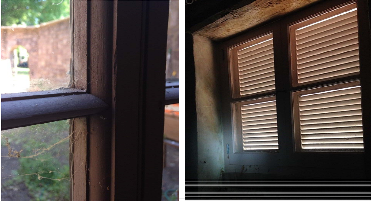
Figure 1.3-11: (Left) The crisp profiles and lack of paint accumulation on the window sashes suggest strongly that they are replacements, likely dating to 1969; (Right) The paired two-light basement casements and the exterior louvered shutters date to 2011.
