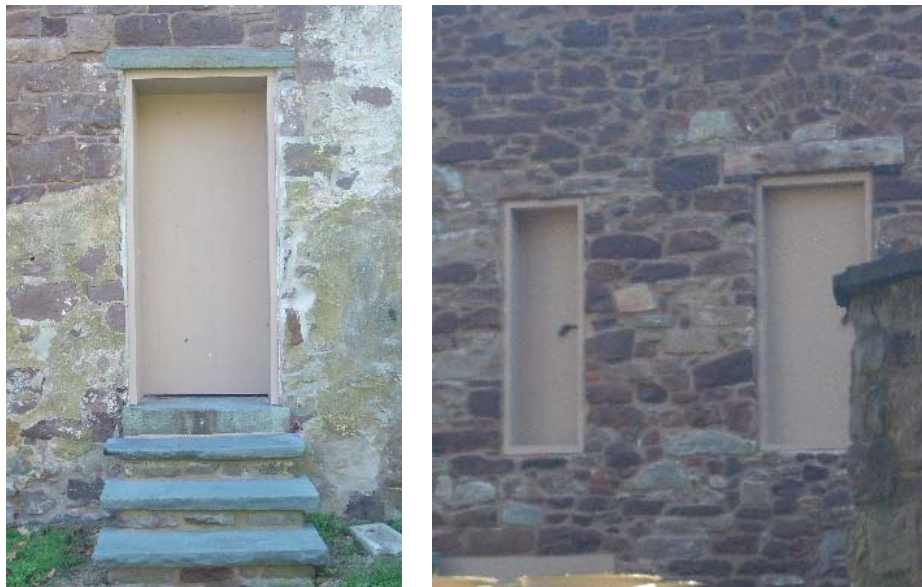
Figure 1.3-10: (Left) The north door opening into the former lock-up area is a later addition. (Right) The two doors on the west elevation access the surviving second-tier jail cells.
