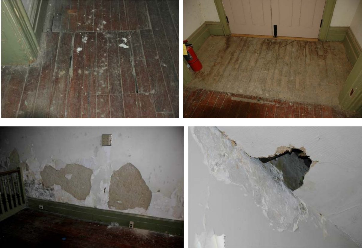
Figure 1.5-25: Detail view of poorly matched patching and damage to individual boards in Room 102 (top left) and detail view of wear and water damage at east vestibule in Room 102 (top left).Detail view of severe water damage to plaster in Room 102 (bottom left) and detail view of plywood ceiling damage in Room 102 (left). Note original wall plaster above the plywood ceiling and damage (bottom right).
