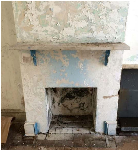
Figure 1.5-47: Detail view of plywood covering in Room 208 (top left). Detail view of damaged and missing plaster in Room 208 (top right). Detail view of fireplace in Room 208 (left).
