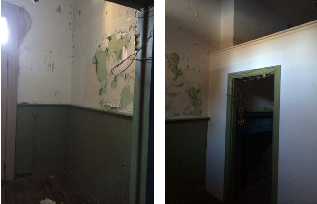
Figure 1.3-31: Views of Room 110 looking northwest from Room 109 (left) and looking northeast (right).
