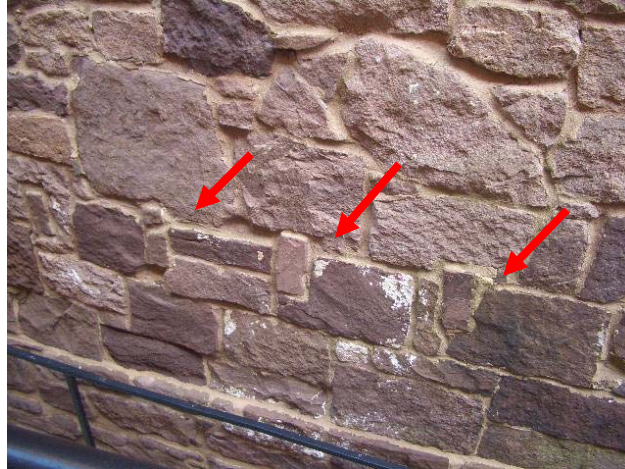
Figure 1.2-28: A series of joist pockets in the south wall appear to mark the location of an exterior platform or stair to access the south door except for the fact that the joists are located above the level of the door sill. The presence of fragments of baseboard nailers indicates this was once an interior surface, probably associated with the courthouse addition. Note also the change in the character of the masonry below the joist level, suggesting this wall was substantially altered.
