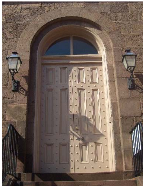
Figure 1.3-8: The main entrance doors are reproductions based on the design of the original doors. The existing transom is likely a replacement. It seems unlikely that a prison would not have had a more secure transom opening.
