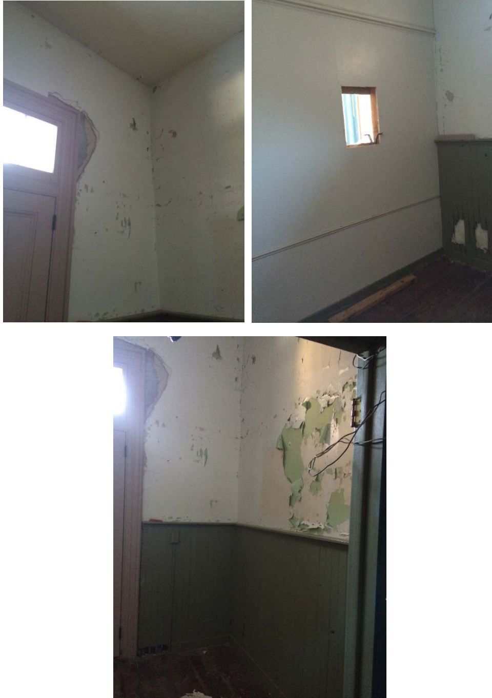
Figure 1.5-33: View of plaster damage at west door (top left) and north wall (bottom) in Room 110. View of penetration in the south drywall partition.
