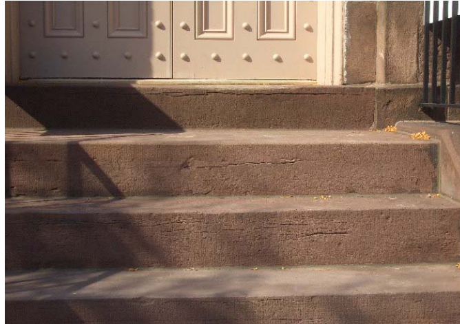
Figure 1.5-7: The front steps of the Sheriff's House consist of large slabs of brownstone. Though the bedding planes are properly oriented, minor delamination is occurring in scattered locations.
