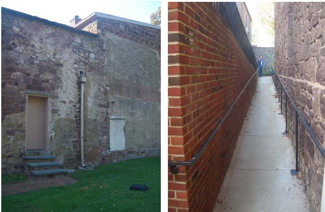
Figure 1.5-1: (Left) Except for the minor depressions located at the downspout discharge points, the grade is relatively flat. (Right) By necessity, the concrete surface of the access ramp located to the south of the building has a neutral slope except at the landing area.
