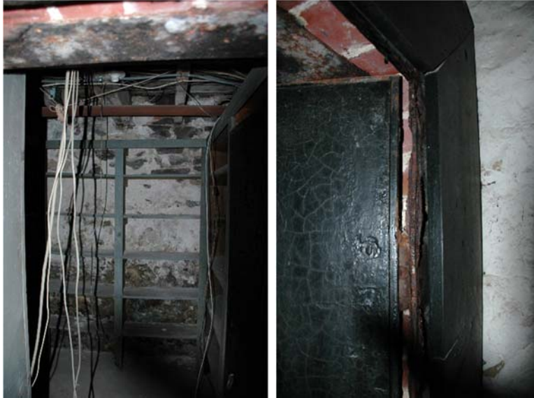
Figure 1.5-20: View of missing plaster and wood shelving at south wall (left) and of rust damage to metal door in the north wall (right) of Room 005.
