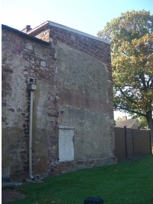
Figure 1.3-5: The rubble masonry seen at the northwest corner of the Sheriff's House retains valuable evidence of the now-demolished prison.
