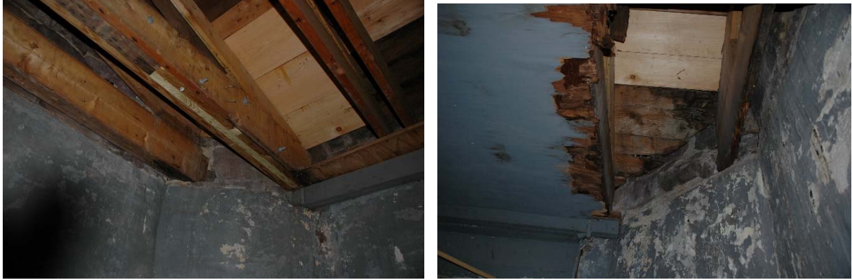
Figure 1.5-37: View of exposed roof framing and damaged plywood ceiling in Room 114.
