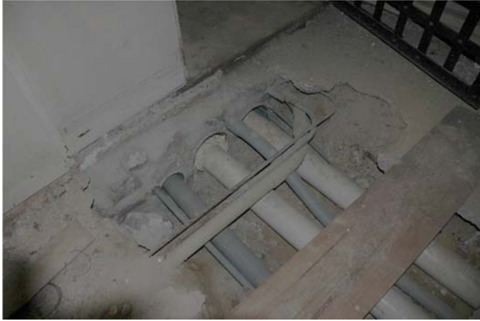
Figure 1.5-34: Detail view of badly damaged floor in Room 111.
