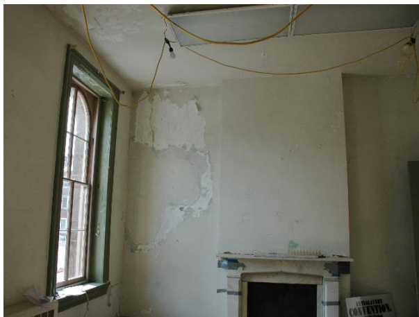
Figure 1.3-24: Views of Room 103 looking east (top) and a detail view of plaster damage at the southeast corner (bottom).
