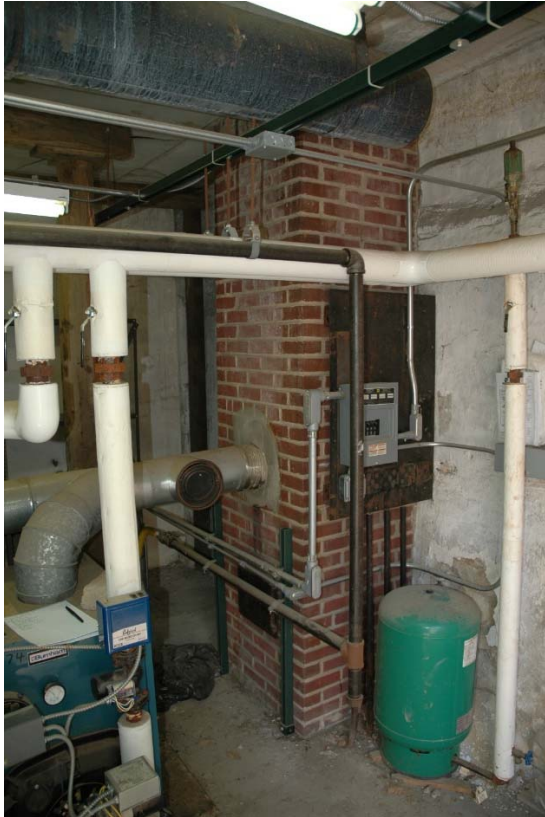
Figure 1.3-36: Views of Room 115 looking southeast at modern brick flue (left) and looking northeast at north wall and mechanical equipment (bottom).
