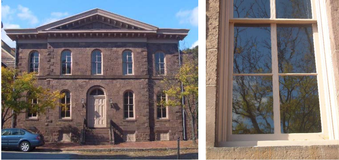
Figure 1.5-14: (Left and Right) The arch-headed windows on the east façade appear to be relatively recent replacements and are in generally good condition. The use of wide vertical muntins with narrow horizontal muntins is somewhat unusual.
