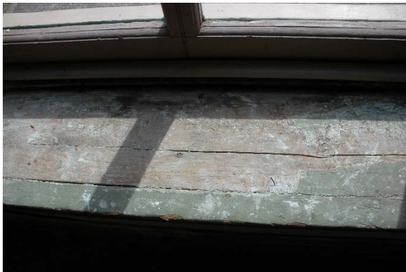
Figure 1.5-22: Detail view of fireplace in Room 101. Note damage at firebox and hearth (top). Detail view of window sill damage in Room 101 (bottom).
