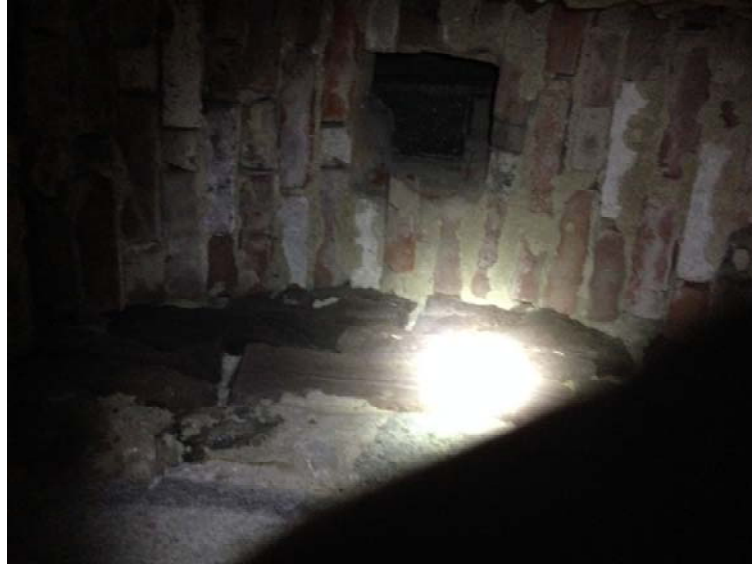
Figure 1.2-60: The brick-vaulted arch in the fireplace foundation located on the north wall of Room 006 has a small flue opening consistent with a coal stove. However, the chimney mass above is truncated at the second-story level.
