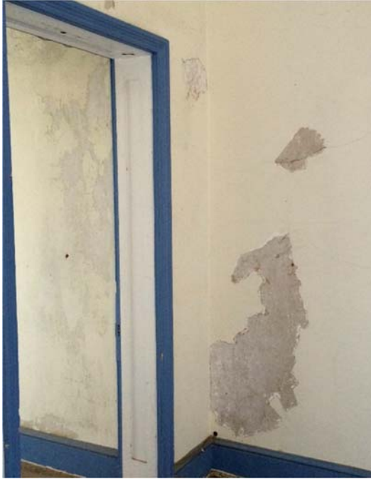
Figure 1.5-42: Detail view of paneled jamb at door to Room 203 from Room 205. Note plaster damage at wall (right).
