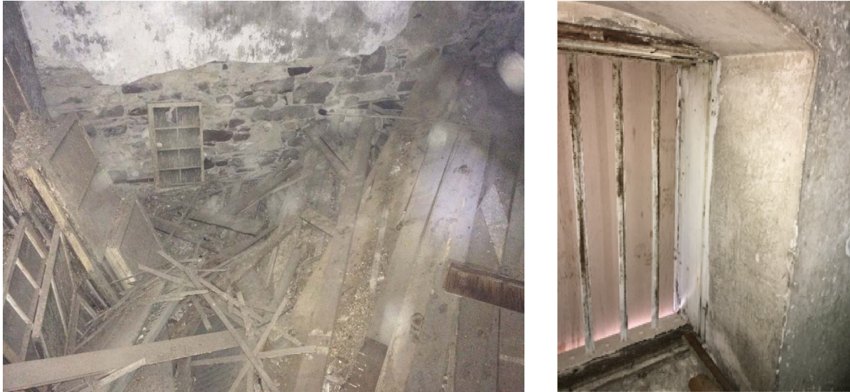
Figure 1.5-49: View of debris on the floor and plaster deterioration at the north wall in Room 211 (left). View of iron bars and deteriorating wood sill and head at Door 2/211 (right).
