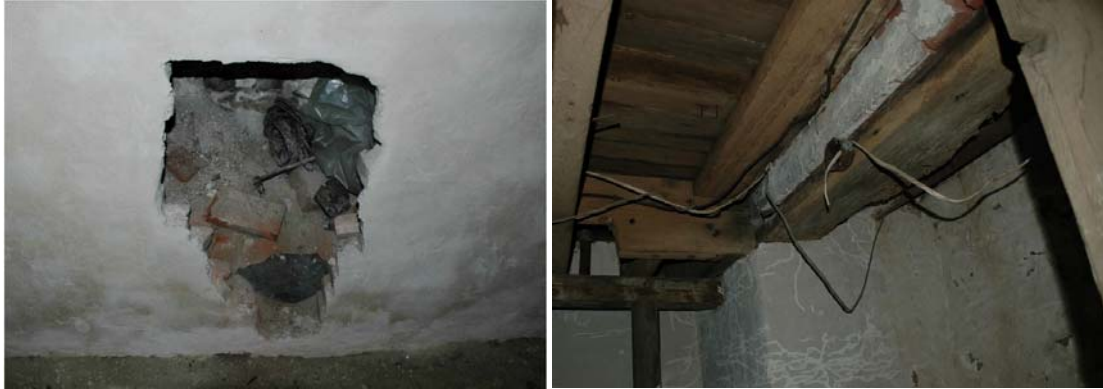
Figure 1.5-21: Area of parging damage/removal at north chimney support in Room 006 (left). Damage/removal appears to have occurred at location of chimney's ash dump. Detail view of deteriorating lintel over exterior wall opening in west wall of Room 006 (right).
