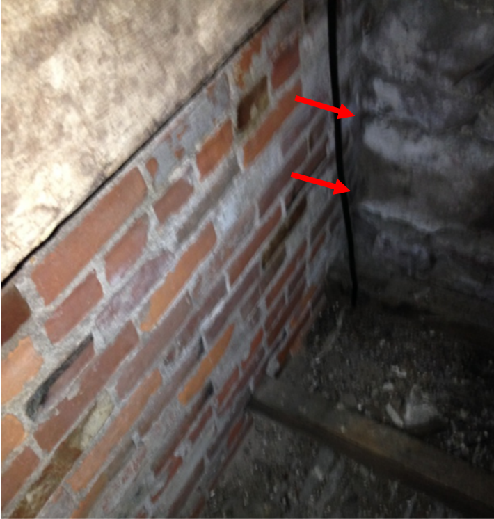
Figure 1.2-22: The brownstone masonry of the south wall appears to have been filled in around the south end of the brick masonry walls enclosing the stair with little attempt to bond the two together.
