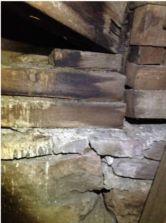
Figure 1.2-23: The north valley beam bears on a pile of scrap wood set on the exterior masonry wall. The contractors made liberal use of recycled materials, presumably to save money.
