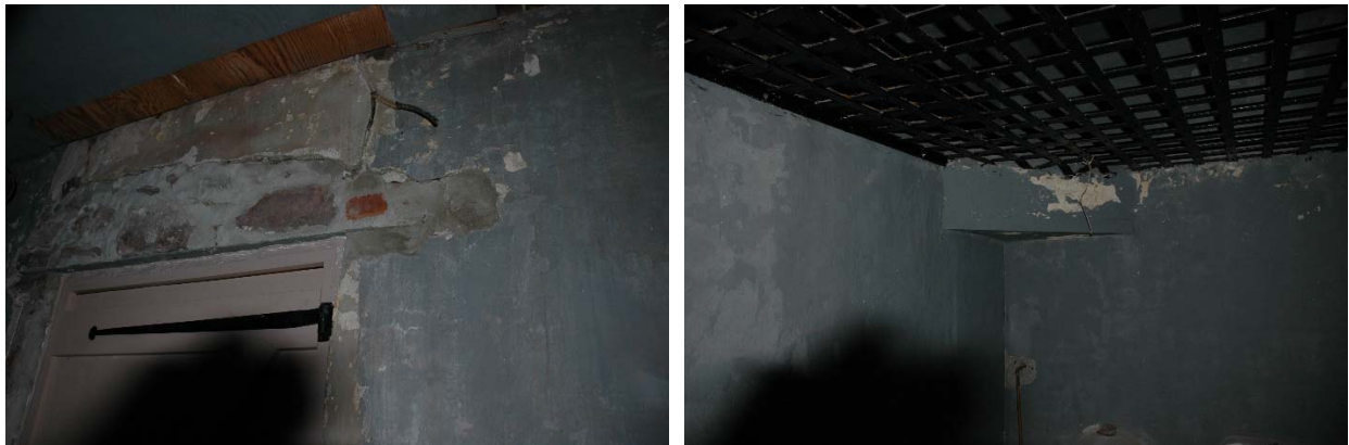
Figure 1.5-38: Detail view of missing plaster where masonry was rebuilt (left). Detail view of cracking at concrete shelf support for cell ceiling (right). Both views in Room 114.
