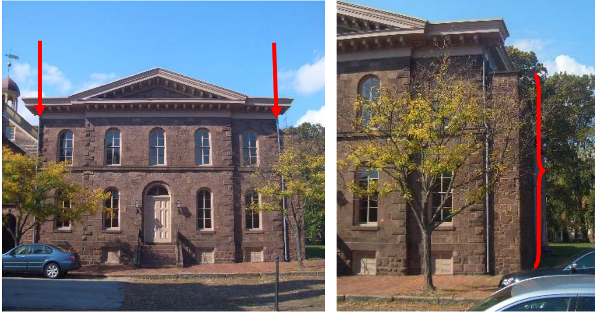
Figure 1.2.18: (Left) The street facade of the Sheriff's House is intended to appear symmetrical with the northeast and southeast corner quoins placed equidistant from the center entrance. (Right) The north end of the building from basement through second floor extends approximately 24 inches farther north in plan.
