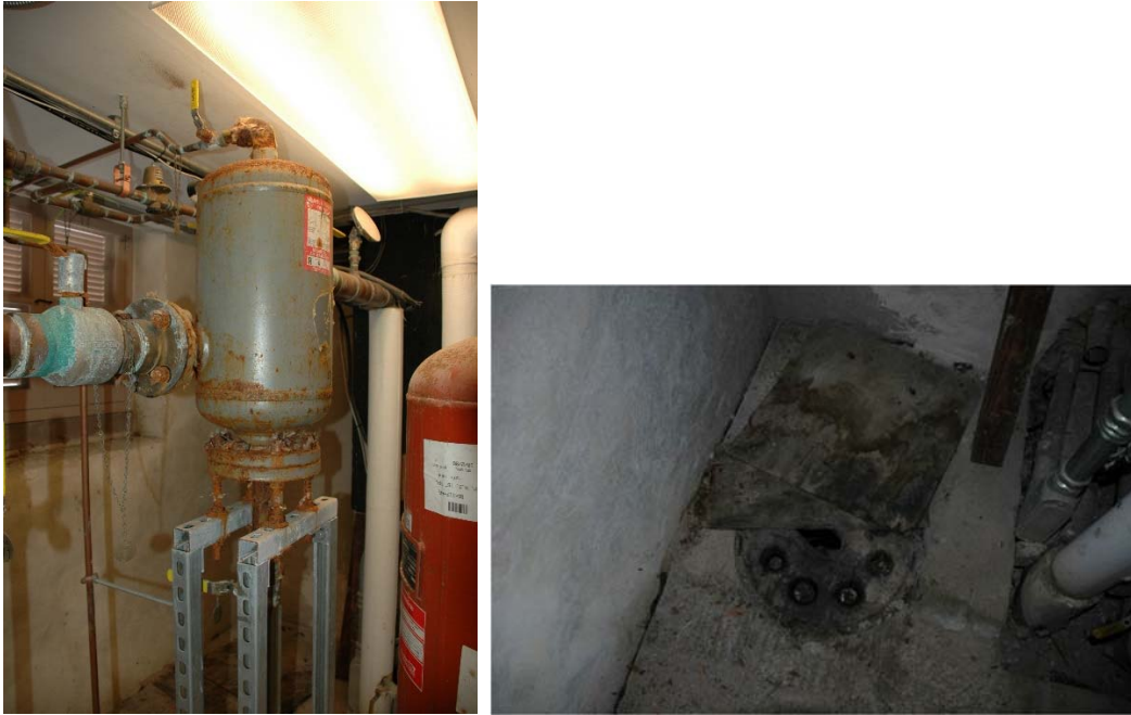
Figure 1.5-18: View of mechanical equipment (left) and floor sump (right) in Room 003.
