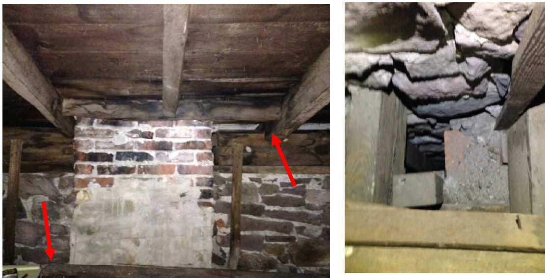
Figure 1.2-34: (Left) View of chimney stack serving fireplaces in Room 103 and 206. Left arrow denotes location of false chase seen in detail at right. Right arrow indicates original width of chimney stack.
