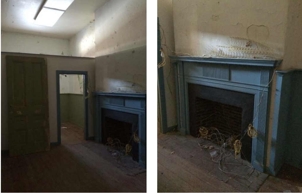
Figure 1.3-30: Views of Room 109 looking northwest (left) and detail view of fireplace at north wall (right).
