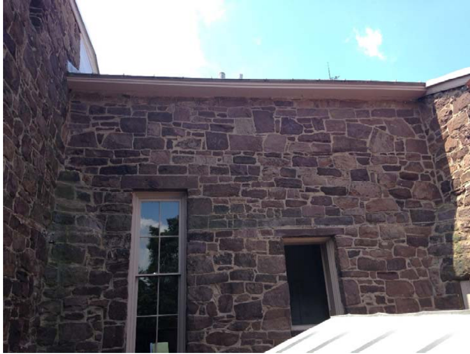
Figure 1.3-14: The second-story windows on the north elevation were installed at different times. The trim at the double-hung window at left does not match the simple trim on the casement window at right. The casement is a later addition.
