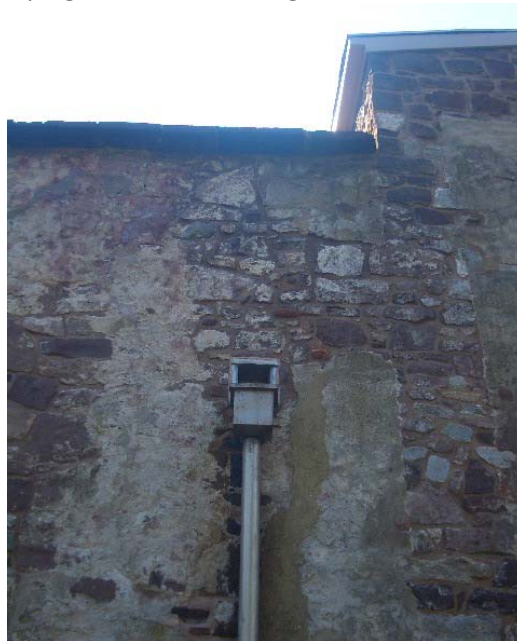
Figure 1.5-8: Rubble stone masonry on the north wall contains significant architectural evidence. Future maintenance repointing should be kept to a minimum to avoid loss of features.
