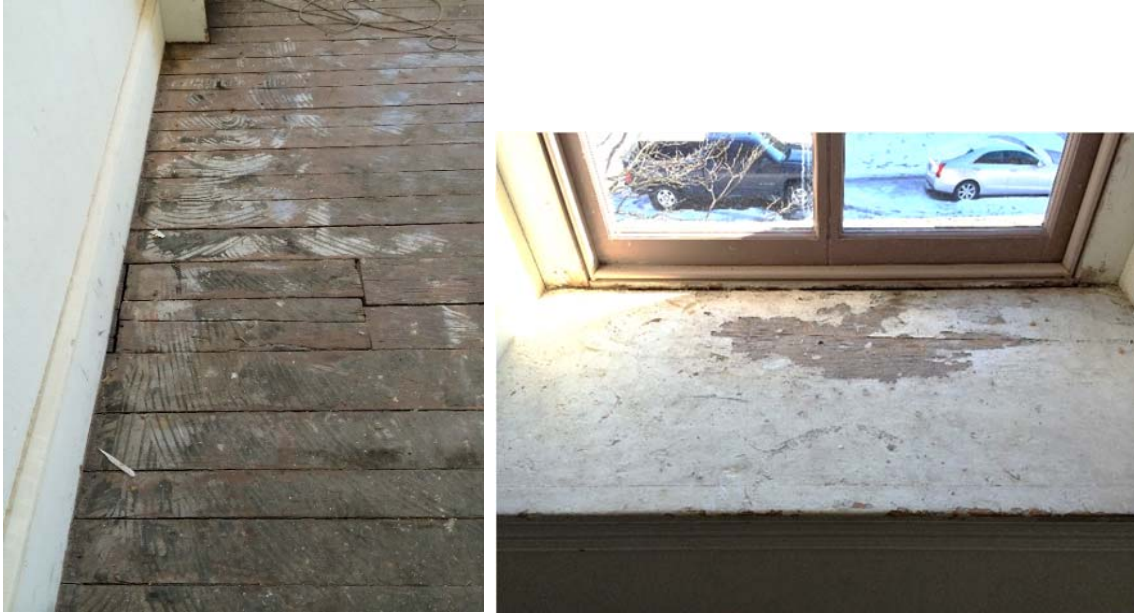
Figure 1.5-41: Detail view of flooring patch in Room 202 (left) Detail view of window stool damage in Room 202 (right).
