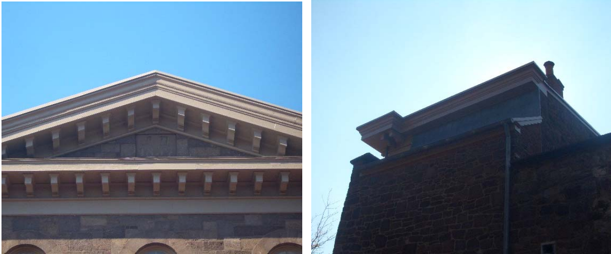
Figure 1.5-9: (Left) Documentary evidence suggests that the modillion cornice has been at least partially replaced. The existing installation, though not inspected at close range, appears to be in good condition. (Right) The modillion cornice transitions to a simpler profiled cornice at the sides of the building.
