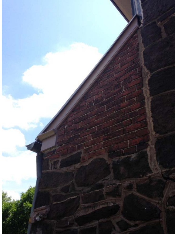
Figure 1.2.19: To accommodate existing walls, the symmetrical main mass of the Sheriff's House appears to have been set just south of center on the foundation of the previous structure, leaving a 24-inch extension at the north end which is truncated to fit behind the adjoining prison yard wall (now removed). Above the height of the prison yard wall, the north wall of the building steps back in line with the main block and is of wood-framed construction rather than masonry.
