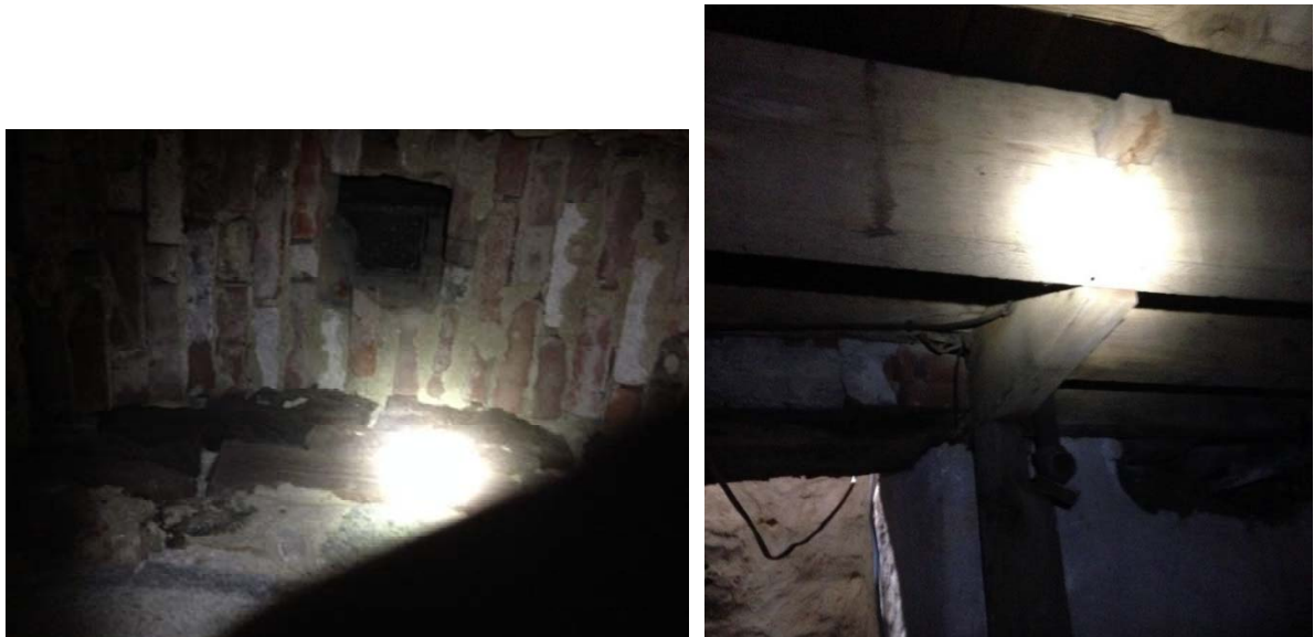
Figure 1.2-47: (Left) Flue opening inside basement fireplace arch in southwest room (Room 006). (Right) Niche in fireplace foundation in basement southwest room (Room 006). The small flue size and a lack of char marks on the plaster inside the arch suggest that a stove was used at this location for heating and/or cooking. (Right) Framed opening for a former exterior basement stair.
