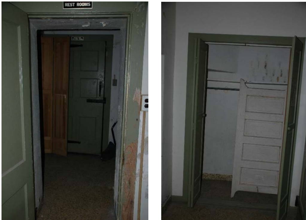
Figure 1.3-33: Views of Room 112 looking south from Room 114 (left) and looking west at closet (right).
