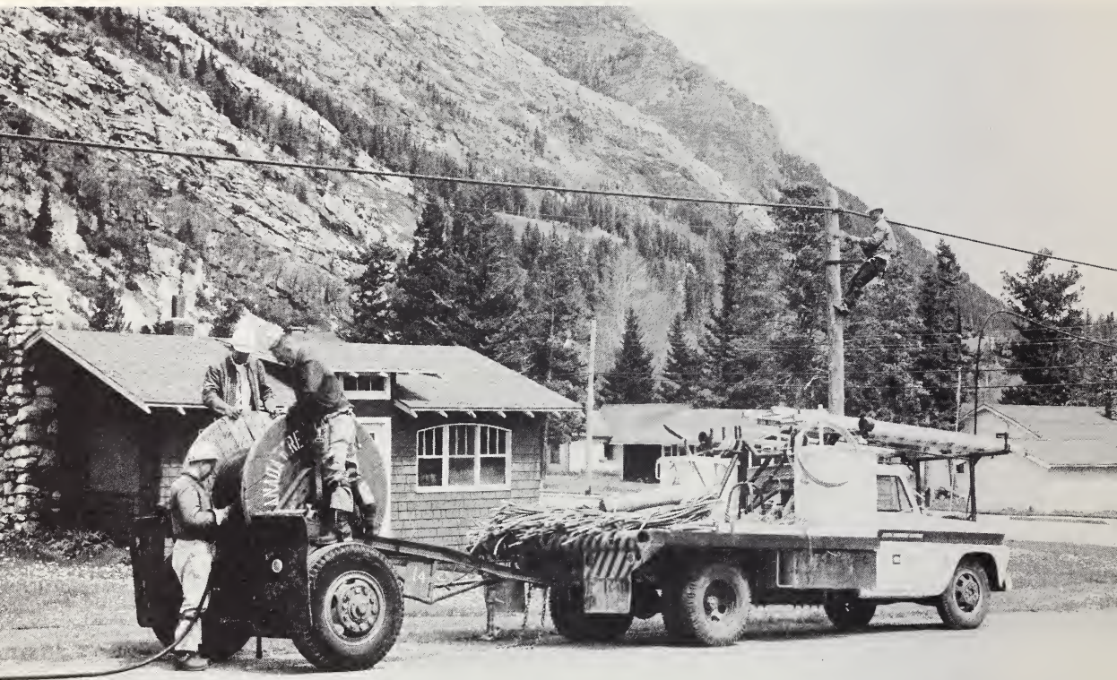
An AGT crew is shown installing exchange cable in Waterton Park. During the year, $1,860,000 was spent on additional cable throughout the Province.
