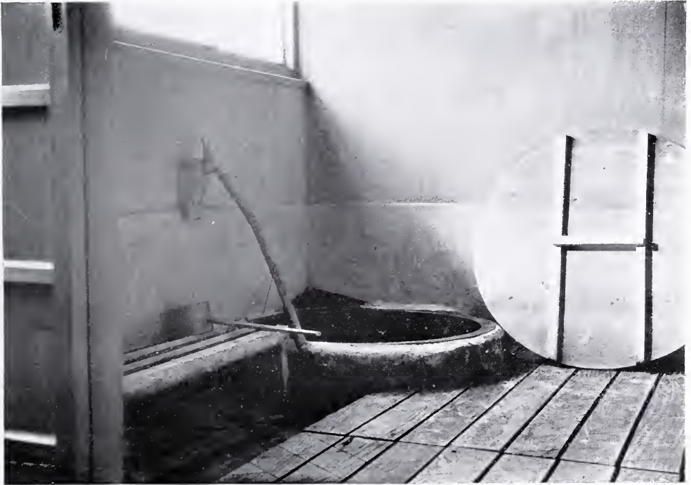
FIG. 23. BATHROOM IN PRIVATE HOUSE.
