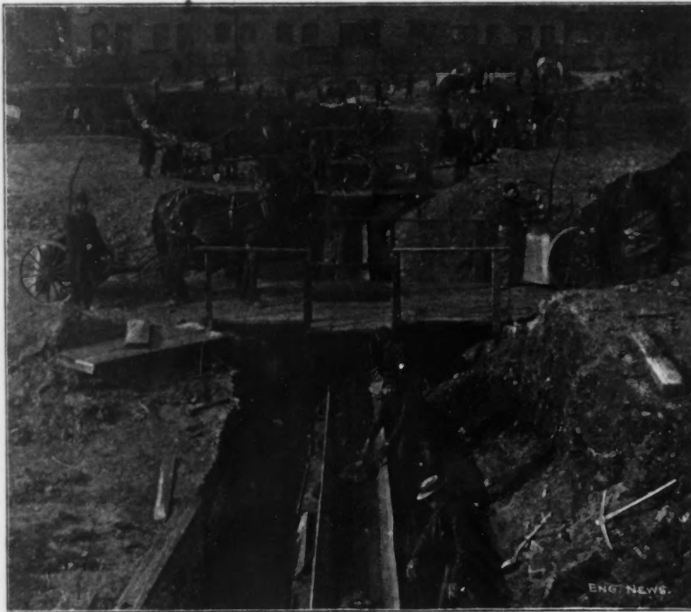
FIG. 1.—GENERAL VIEW OF BELT CONVEYOR PLANT FOR HANDLING EXCAVATED MATERIAL IN CONSTRUCTING A LARGE POWER HOUSE FOUNDATION.
