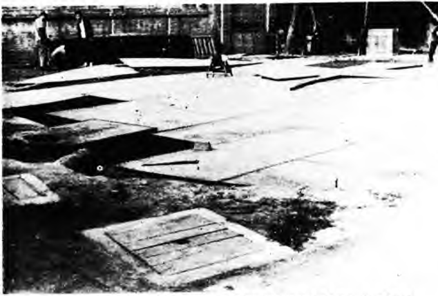
BOTTOM PLATES OF OLD SETTLING TANK BEING DISMANTLED FOR MAKING CASING OF NEW WELL.
