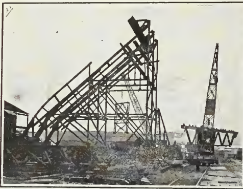
Illustrations show part of an incline gantry for the Delagoa Bay Coaling Plant, under construction.
