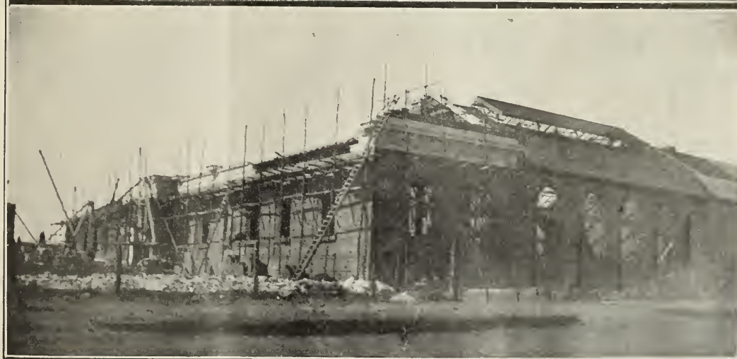
Two Views of the New Mint, under construction at Pretoria. An article on the Mint appears elsewhere in this issue.
