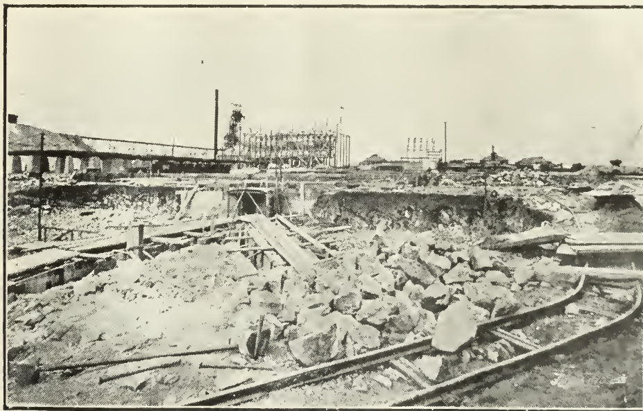
Construction work in progress on a big Rand Mine. A photo of the more prosperous times of a few years ago which we all should like to see return.
