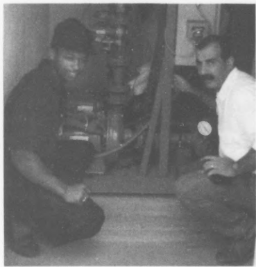
Ricardo Filipe Cardiga, right, inspects water pumping equipment.
