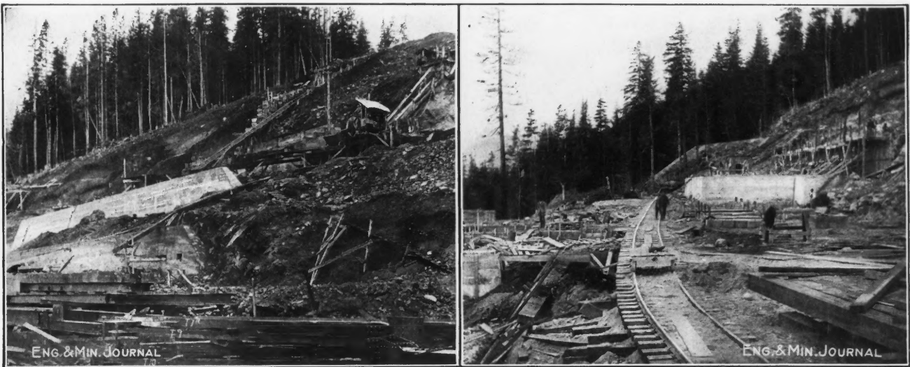
THE HIDDEN CREEK MAIN SMELTER BUILDING, DUST CHAMBER, FLUE AND STACK SITES View at left as it appeared July 11; at right as of May 27.
